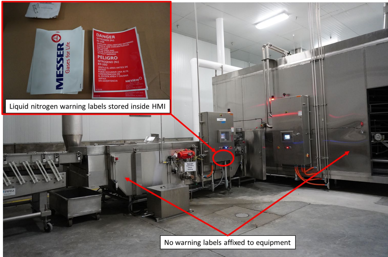
Figure 27. Liquid nitrogen warning labels were located inside the HMI and were not affixed to equipment. (Credit: CSB)
