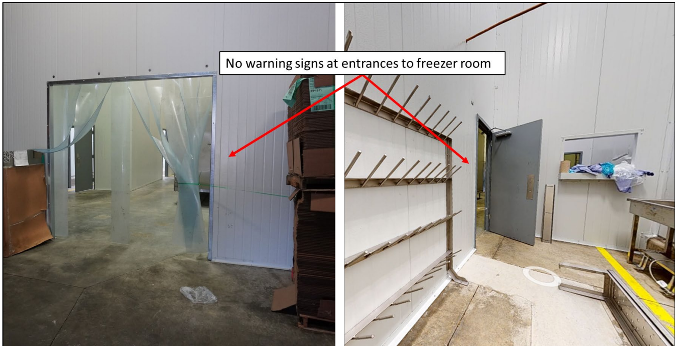
Figure 26. Lack of warning signs for the presence of liquid nitrogen and asphyxiation hazard at the entrance to the freezer room from the loading dock (left) and clean room (right). (Credit: CSB and Messer)
