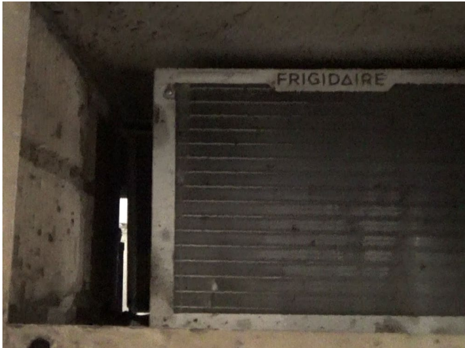
Figure 21. Wall-Mounted Air Conditioner. This photo, taken from outside of the PPE Room, shows an opening to the inside of the PPE Room. (Credit: CSB)
