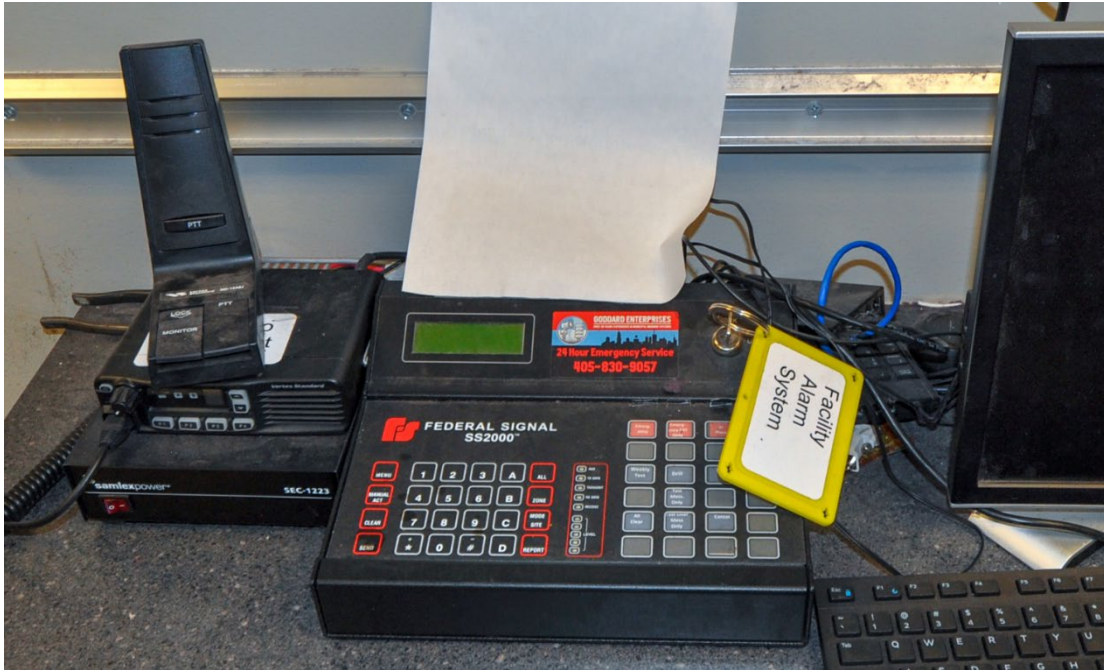
Figure 22. Base Station for Facility Alarm System. (Credit: CSB)
