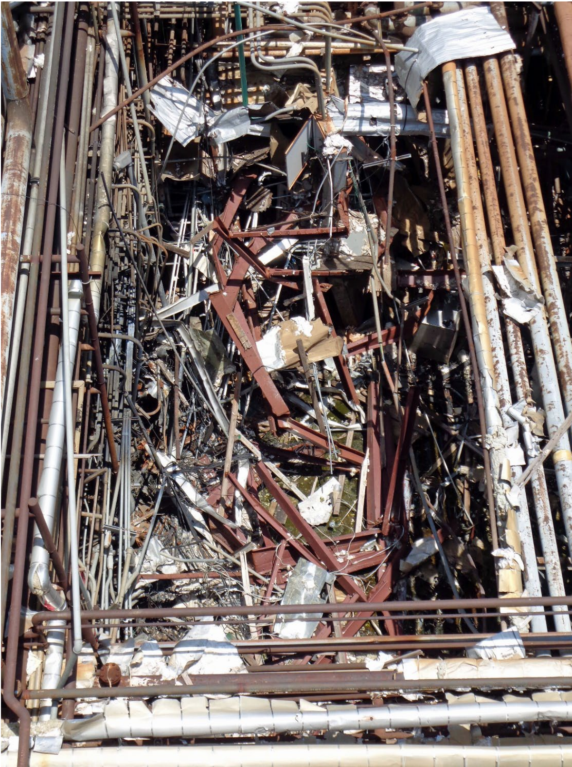
Figure 15. R2 Building (Top View). This photo, taken from the top of adjacent equipment, shows the post-incident condition of the R2 Building. (Credit: CSB)
