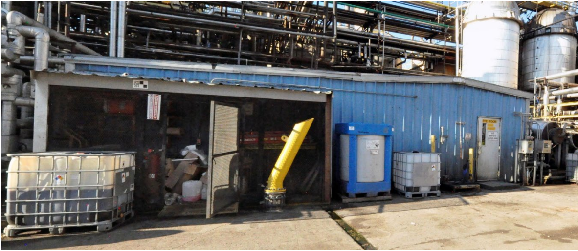
Figure 7. PPE Room. This photo shows the former Reaction 1 Control Room that KMCO converted to store PPE. The construction of the former Reaction 2 Control Room was similar to this building. (Credit: CSB)
