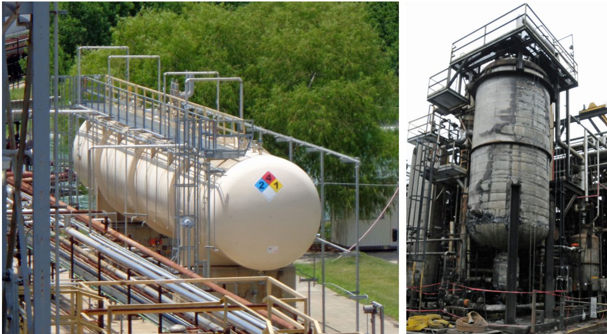
Figure 2. Post-Incident Photos of KMCO’s Isobutylene Storage Tank (left) and Batch Reactor System (right). (Credit: CSB)
