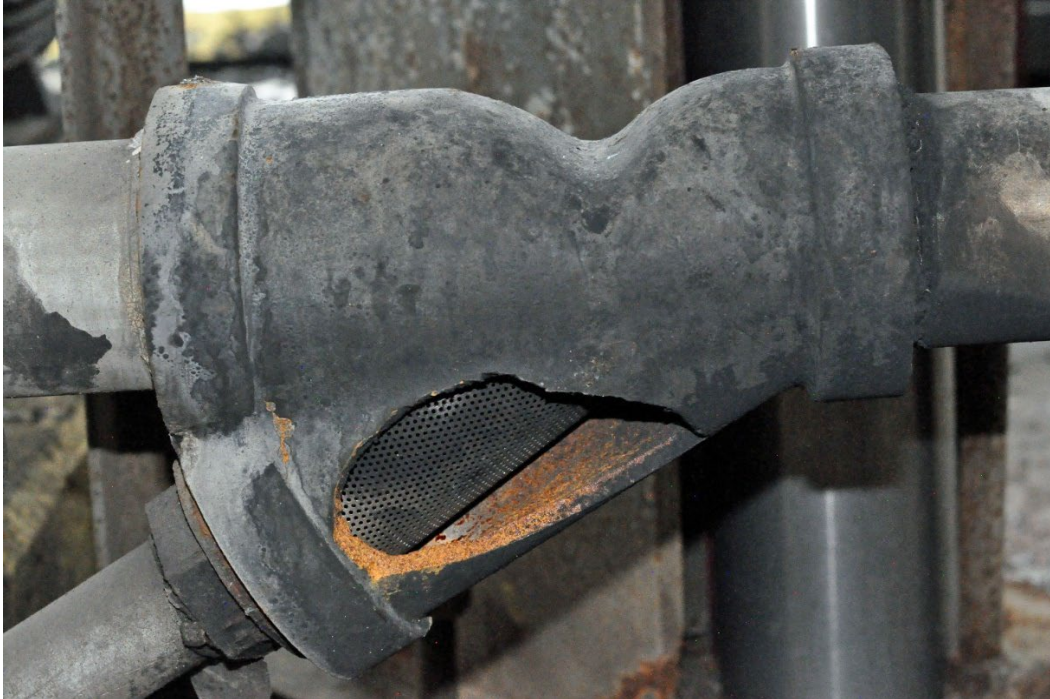
Figure 17. Y-Strainer. This photo shows the west side of the failed y-strainer involved in the April 2, 2019, incident. (Credit: CSB)
