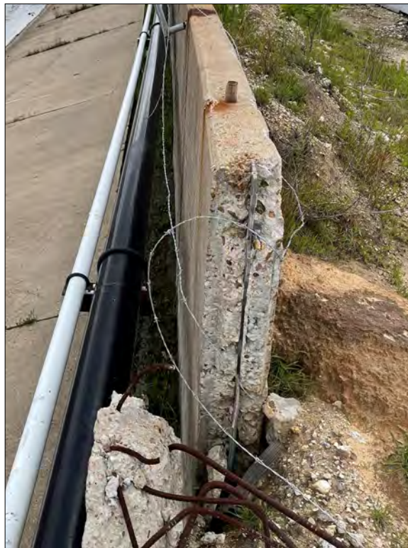
Photo 14: Torn waterstop and displaced wall. Upper section of wall that was displaced has been partially demolished during remediation efforts.
