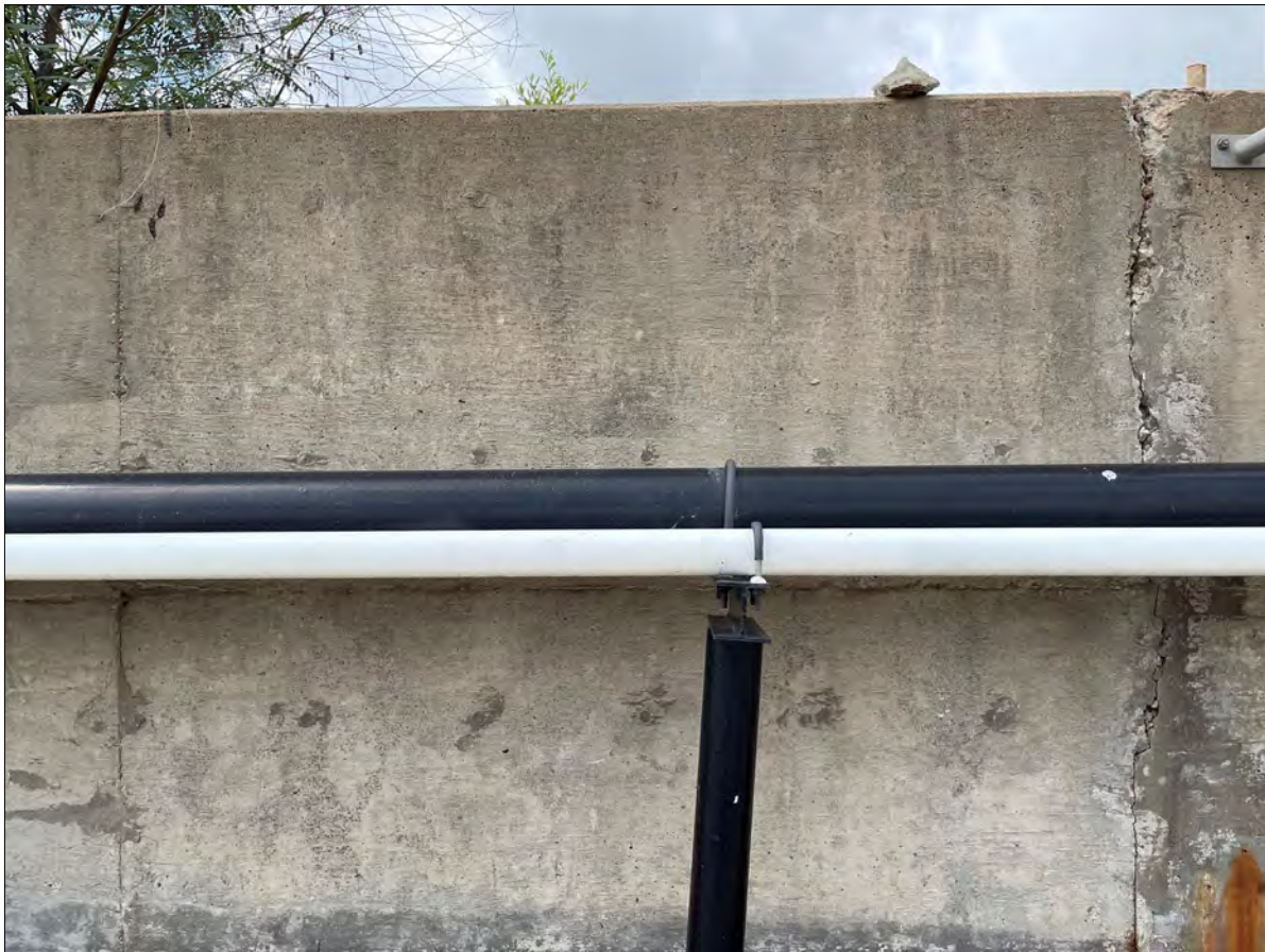
Photo 12: North concrete retaining wall, outside face. Form tie marks on wall
