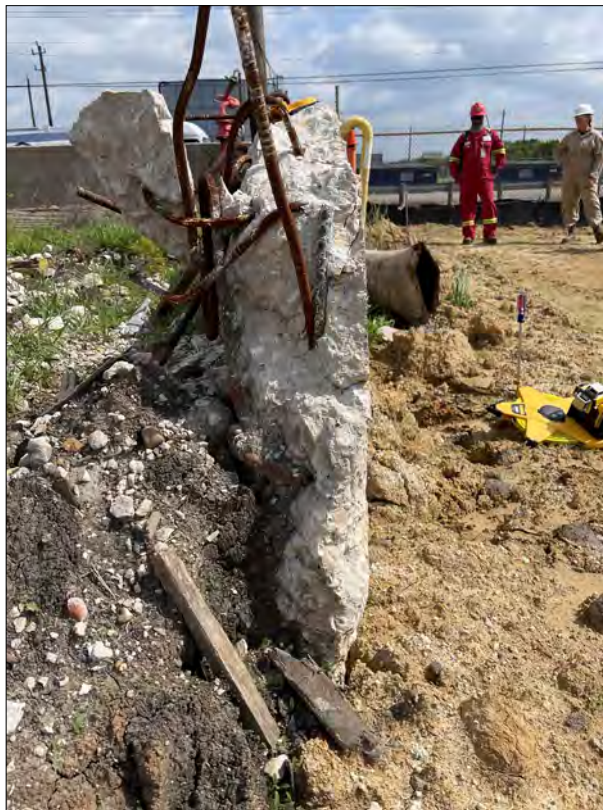
Photo 11: Exposed reinforcement at a section of the east containment wall where the wall was removed during remediation efforts
