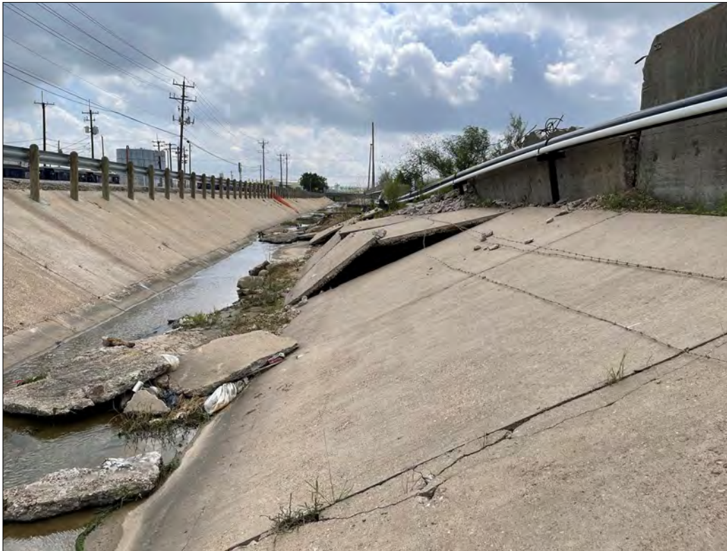
Photo 16: Damaged Section of Drainage Ditch, looking east
