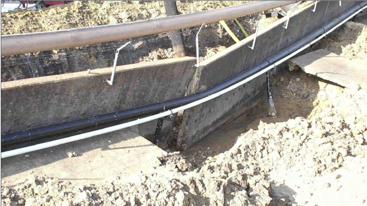
Photo 9: Close-up photo of containment wall breach provided by CSB 17
