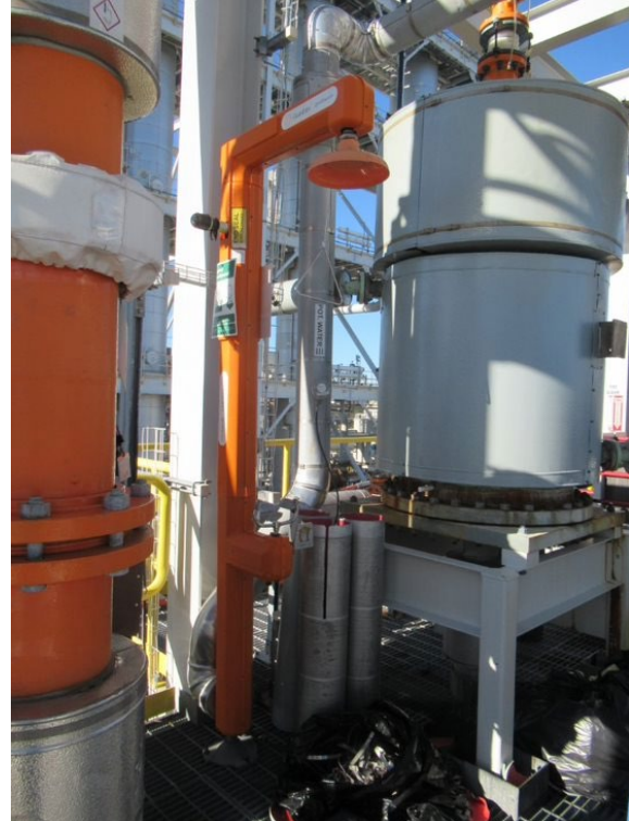
Figure 5. Fifth-floor safety shower. (Credit: CSB)
