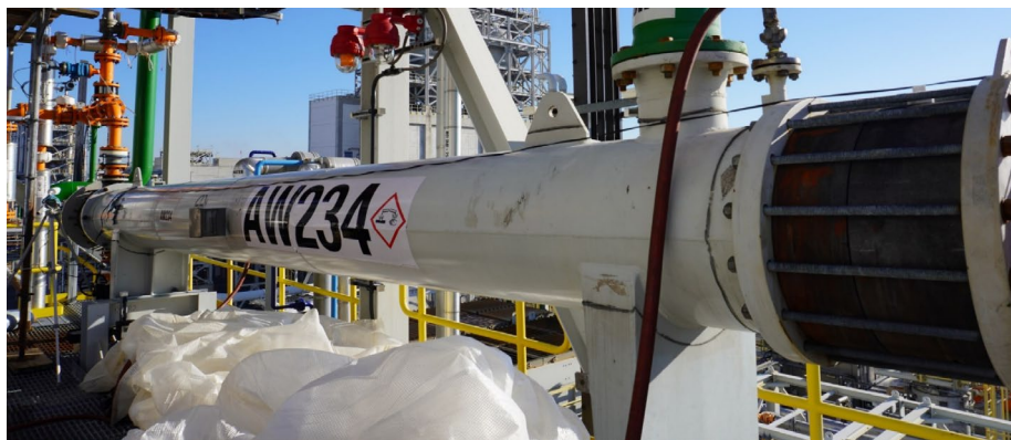
Figure 1. Heat exchanger AW234. (Credit: CSB)
