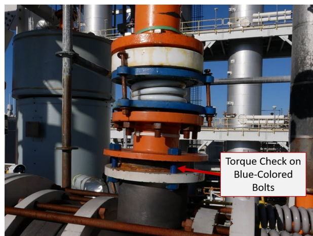
Figure 9. Torque check location. A Jake Marshall employee was checking the bolts connecting the graphite flange when the release occurred. (Credit: CSB)
