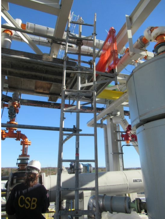
Figure 4. Scaffolding located near the release obstructing movement on the platform. (Credit: CSB)
