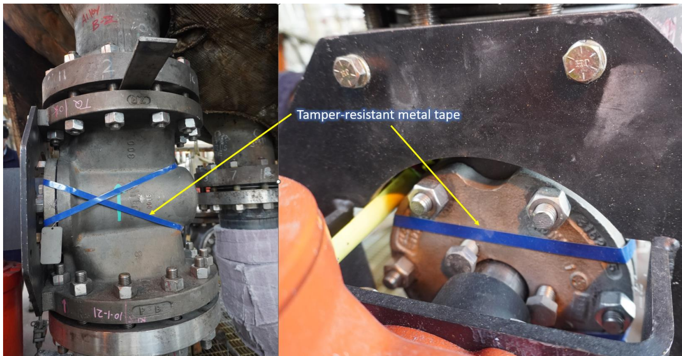
Figure 11. Example of tamper-resistant mechanism incorporated by LyondellBasell. (Credit: CSB)
