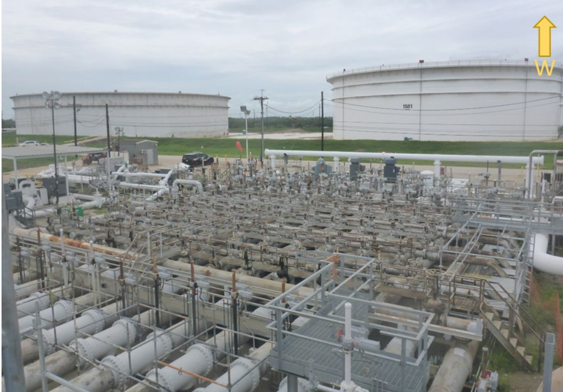
Figure 2. View of central manifold (west facing view). (Credit: CSB)
