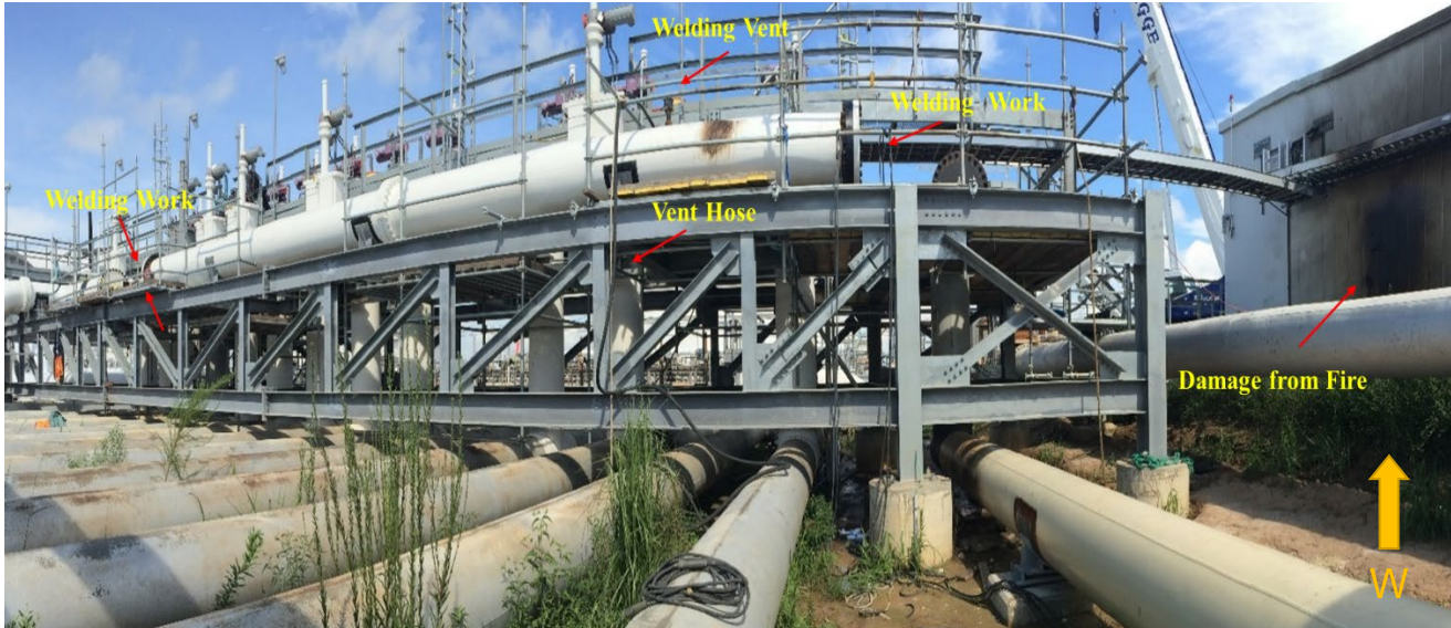
Figure 17. West-facing view of the section of piping where welding work was ongoing (on the north end) at the time of the incident. (Credit: CSB)
