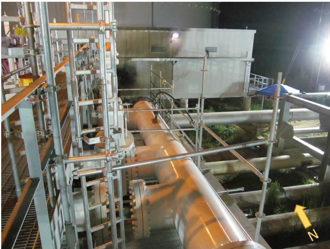
Figure 16. Piping segment where flash fire and explosion occurred. (Credit: CSB)
