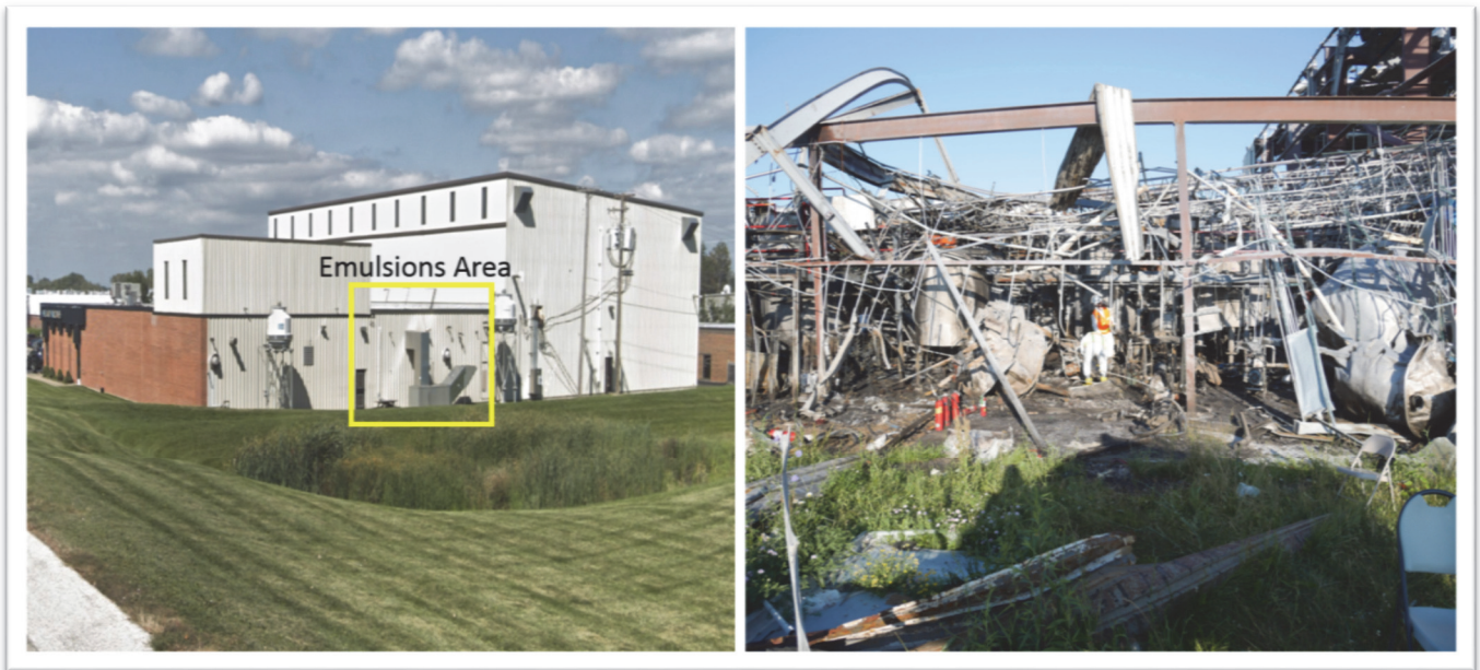
Figure 7. Emulsions Area. On the left, photo of location of the emulsions area prior to the incident. On the right, photo of the emulsions area post-incident. (Source: Google Maps (left); CSB (right)).
