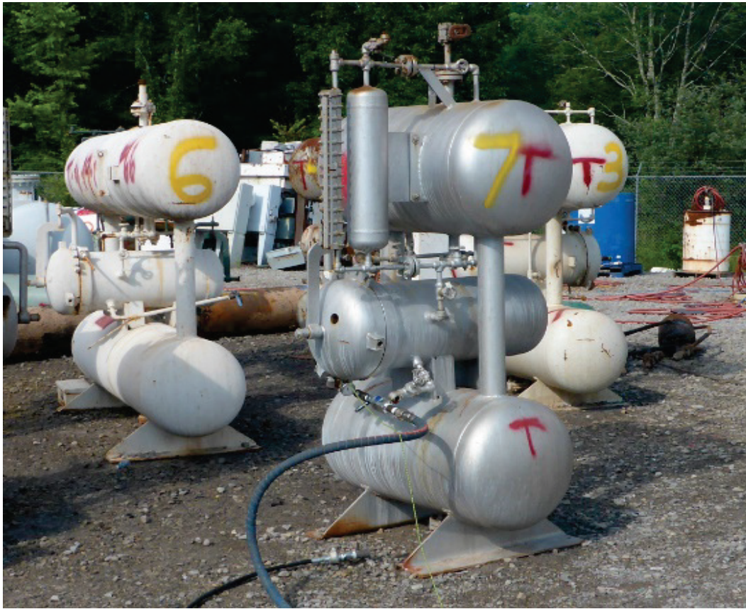
Figure 14. MP Odorizer Before June 20, 2017 Explosion. This pre-incident photo shows the MP odorizer and equipment connections that SPSI workers were using to drain liquid when the June 20, 2017 explosion occurred. a (Credit: CSB).
