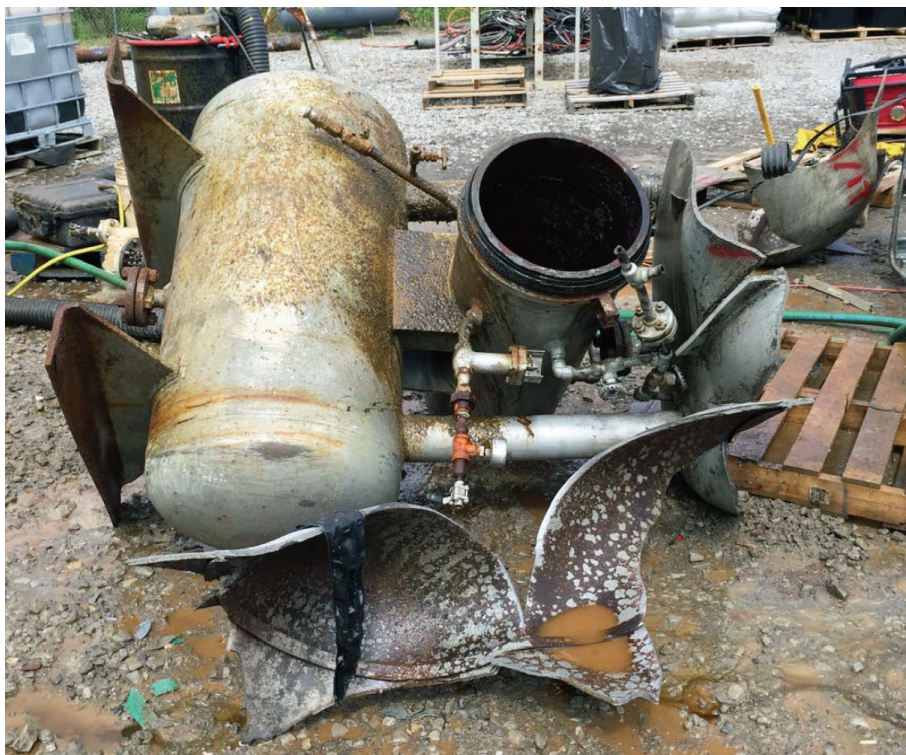
Figure 10. MP Odorizer That Exploded on May 24, 2017. This photo shows the failed MP odorizer from the May 24, 2017, explosion. (Credit: MRR).
