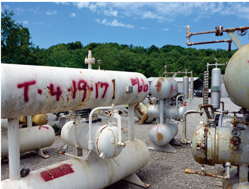
Figure 7. Treatment Status. This photo shows how MRR technicians used red spray paint to record the date the MP was chemically treated, April 19, 2017. (Credit: CSB).
