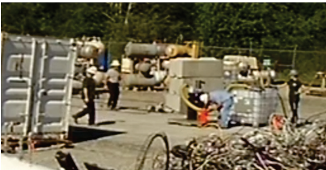
Figure 18. Concrete Barriers. This surveillance video image from June 20, 2017 at 9:56 a.m., shows only one of four SPSI workers positioned behind the concrete barrier. Two other concrete barriers were placed, but they are outside the view of this surveillance camera (Credit: MRR).
