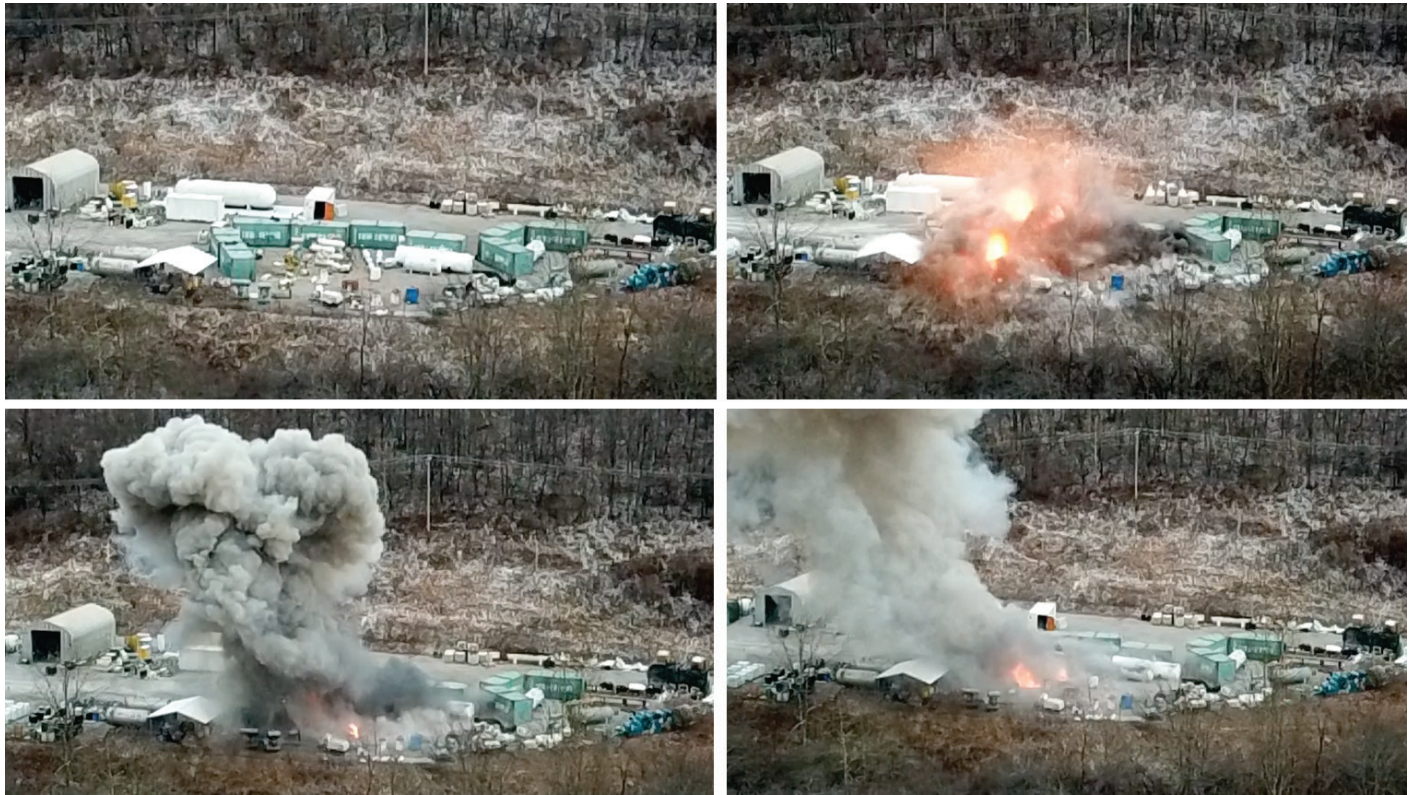
Figure 19. Explosive Venting. These drone video images show the explosive venting used to cut holes in a group of MP vessels to drain the vessels while minimizing risk to people. The bottom right image shows a fire that erupted from flammable liquids that drained from some of the MP vessels. (Credit: MRR).
