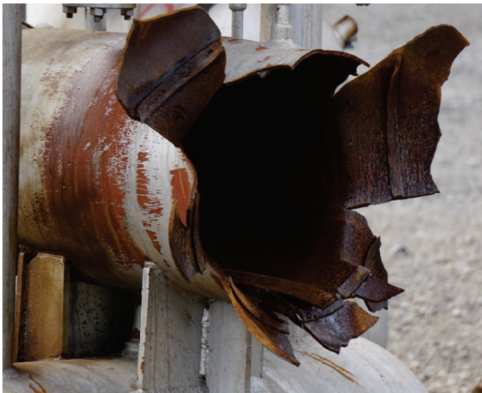
Figure 17. Ruptured MP Odorizer Middle Chamber from June 20, 2017, Incident. This photo shows the post-incident condition of the rounded end of the middle chamber that ruptured in the June 20, 2017, explosion. (Credit: SPSI).
