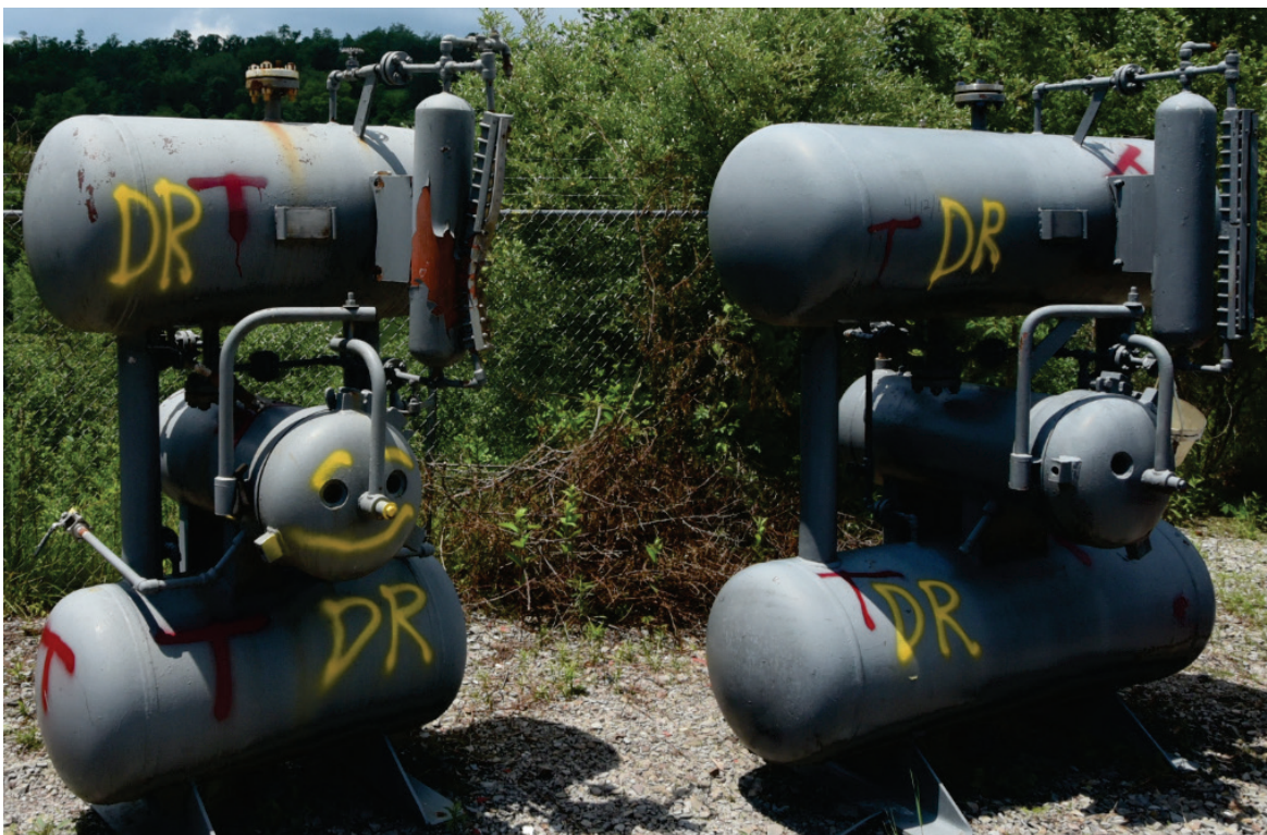
Figure 8. Drained Status. This photo shows how MRR technicians spray painted odorizer equipment with a “D” or a “DR” for drained (in yellow) after they drained the sodium hypochlorite treatment solution from the odorization equipment. (Credit: CSB).
