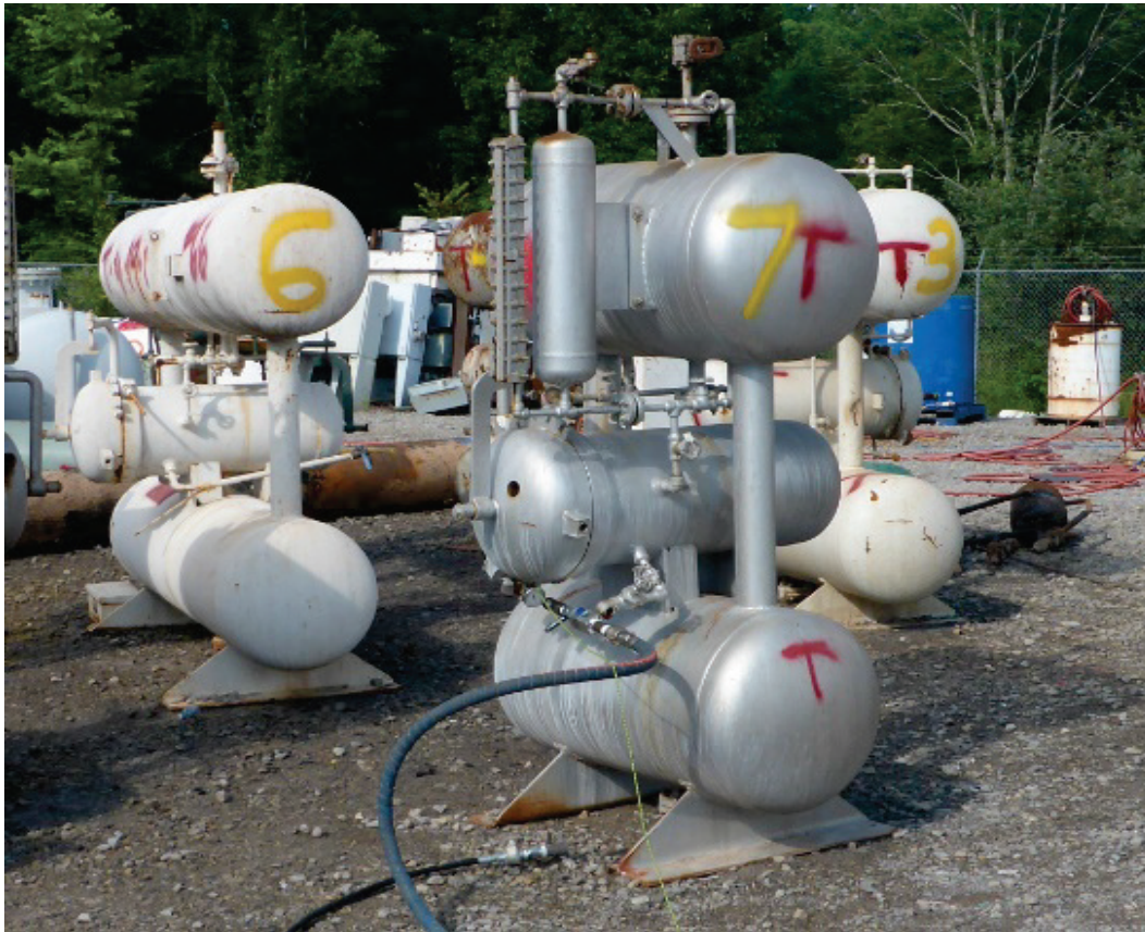
Figure 14. MP Odorizer Before June 20, 2017 Explosion. This pre-incident photo shows the MP odorizer and equipment connections that SPSI workers were using to drain liquid when the June 20, 2017 explosion occurred. a (Credit: CSB).
