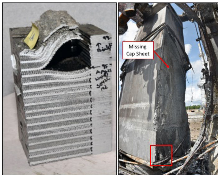
Figure 21. Bulge observed in the ACSR that affected layers 95 through 99 (left). The bulge is on the northeast bottom corner of the exchanger in the area of the missing cap sheet and attachment plate (red box, right). Also shown in the image on the right is the place where the cap sheet is missing from the exchanger.
