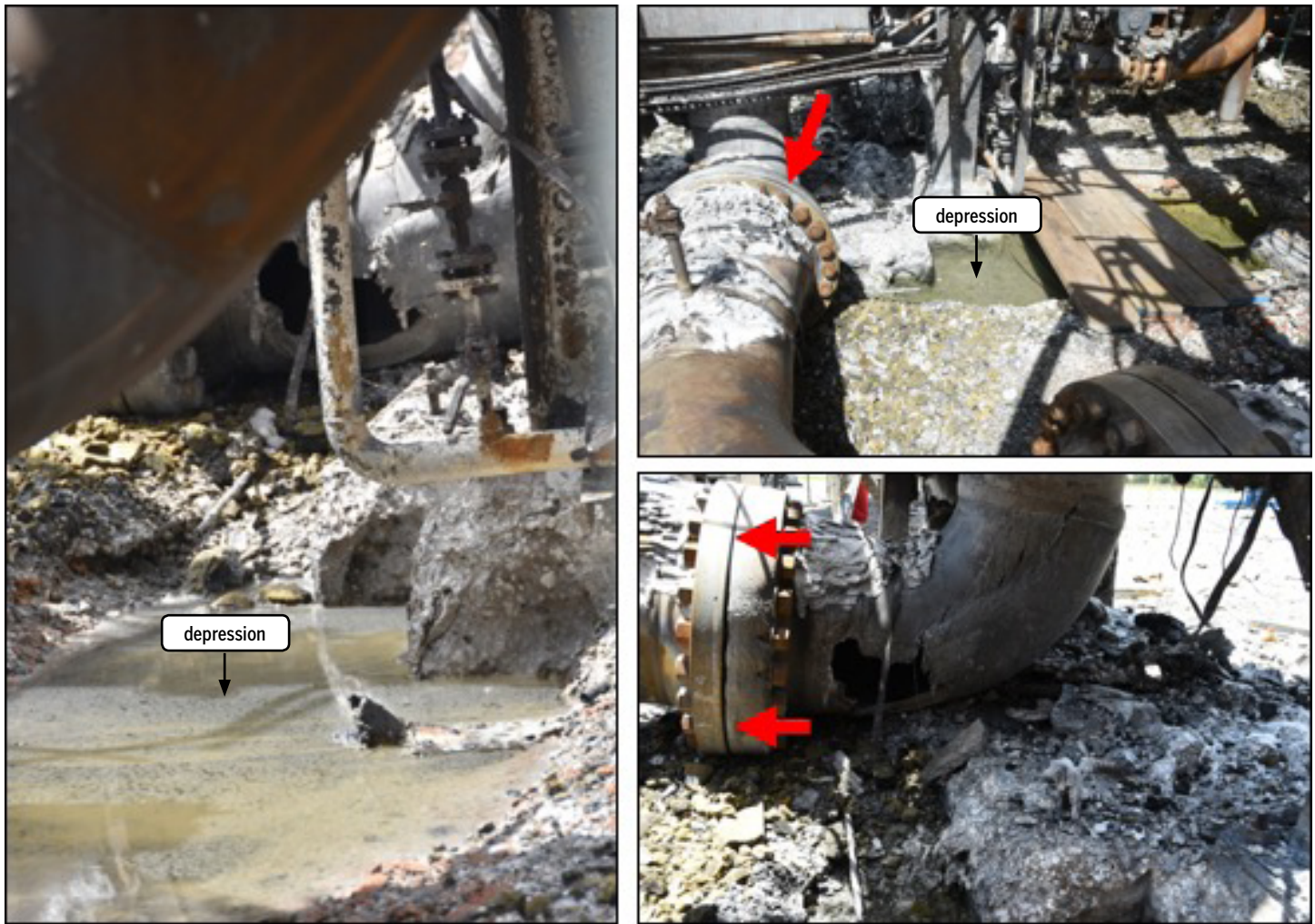
Figure 47. Post-incident examination of the area revealed a large depression in the ground (left and upper right images). The breach visible in the lower right image lines up with the depression in the ground. Red arrows point out the B-inlet flange.
