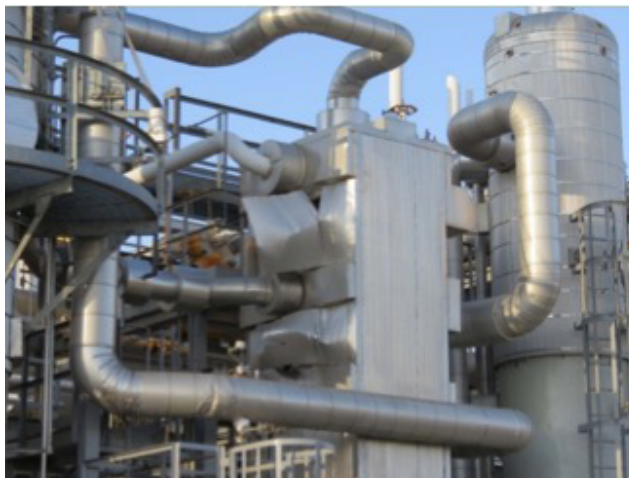
Figure 24. Ruptured cold side reboiler at Enterprise's Chaco gas plant, showing the exchanger still covered in insulation. (Credit: Chart Industries)
