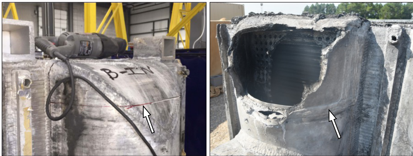
Figure 45. The B-inlet header on the ACSR is marked for cutting during the September 2015 repair (left, white arrow). The breach found in the B-inlet header post-incident partially followed the new weld (right, white arrow).
