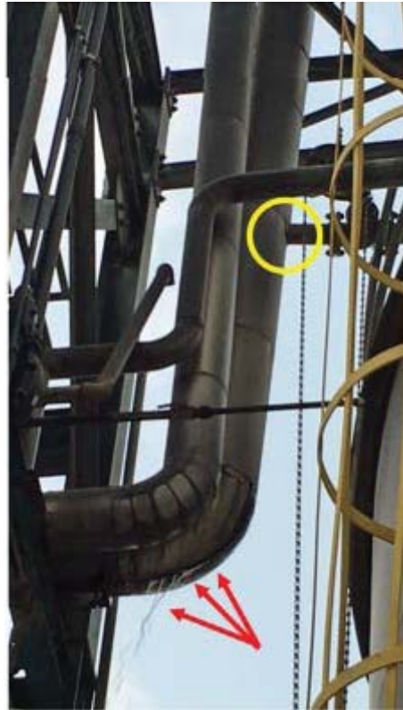
Figure 12. Pre-Incident Photograph of the Water Leak. The water piping (yellow circle) had cracked at the connection point between the eight-inch vertical water piping and the three-inch horizontal piping entering the foul condensate tank. Water was leaking from the crack (red arrows). Photograph: PCA.
