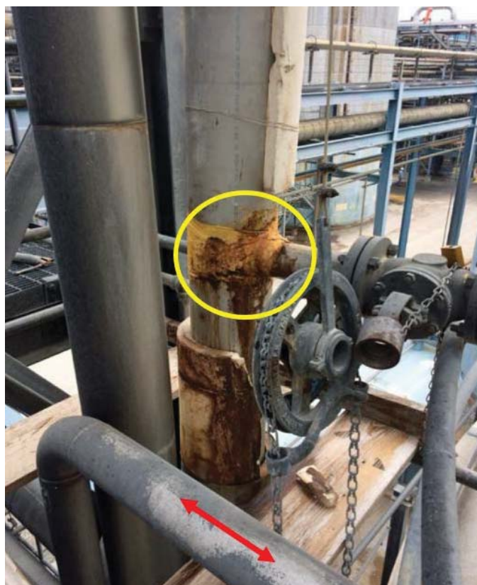
Figure 11. Pre-incident Photograph of the Cracked Three-inch Piping Connection on the Eight-inch Water Piping (yellow circle). This photograph shows a temporary repair to slow the leak, installed in October 2016. Witnesses stated that workers repaired this crack before the explosion. Workers disconnected the water piping from the valve (just to the right of the yellow circle) to create an air gap and to separate the repair area from the foul condensate tank. The red arrow shows the adjacent vent piping from the foul condensate tank to the CNGC system. The valve on the foul condensate side of the air gap, which was never located, was reportedly closed leading up to the incident. The vapor inside the foul condensate tank and the vent piping likely contained an explosive mixture of NCG and air when this repair work took place. Photograph: PCA.
