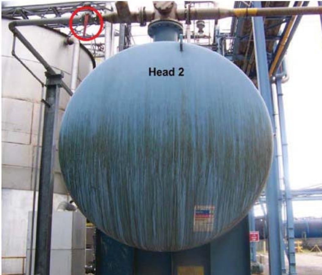
Figure 21. Closed Valve on the Piping from the Foul Condensate Weir to the Turpentine Recovery System. This photograph from the mill's 2010 inspection file shows that the valve is in the closed position. Post-incident, this valve also was found in the closed position. The CSB learned that the PCA DeRidder mill had not used the foul condensate tank's weir system to remove turpentine. Photograph: PCA.
