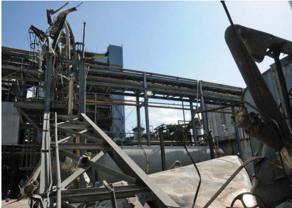
Figure 10. Photograph Showing Explosion Damage at the PCA DeRidder Mill in DeRidder, Louisiana. The bottom right corner of the photograph shows the foul condensate tank's base upside-down. The explosion separated the tank from its base. Photograph: CSB.
