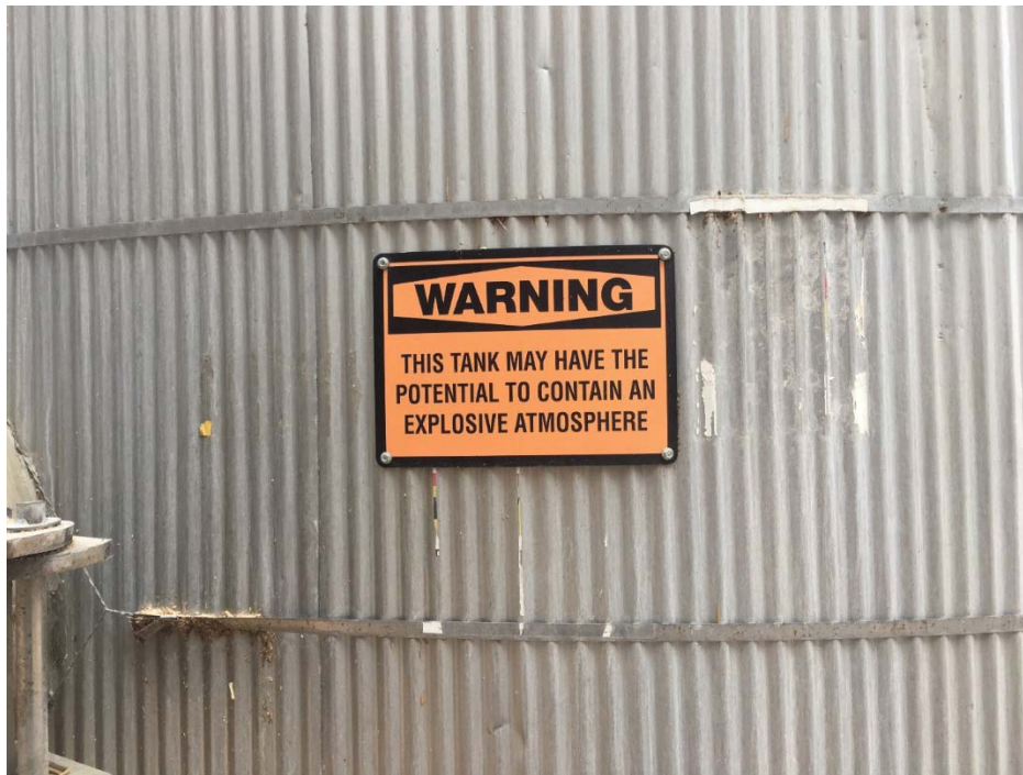
Figure 44. Post-Incident Warning Label. This warning label is intended to inform personnel of the potential hazards associated with a flammable atmosphere inside a vessel. Photograph: PCA.
