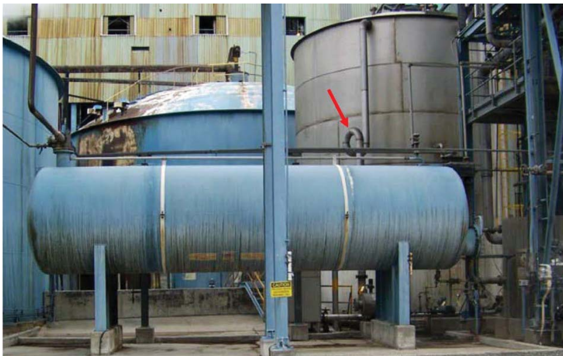
Figure 29. Pre-Incident Photograph Showing Overflow Seal Leg. This pre-incident photograph shows the overflow seal leg on the foul condensate tank (red arrow). Photograph: PCA.
