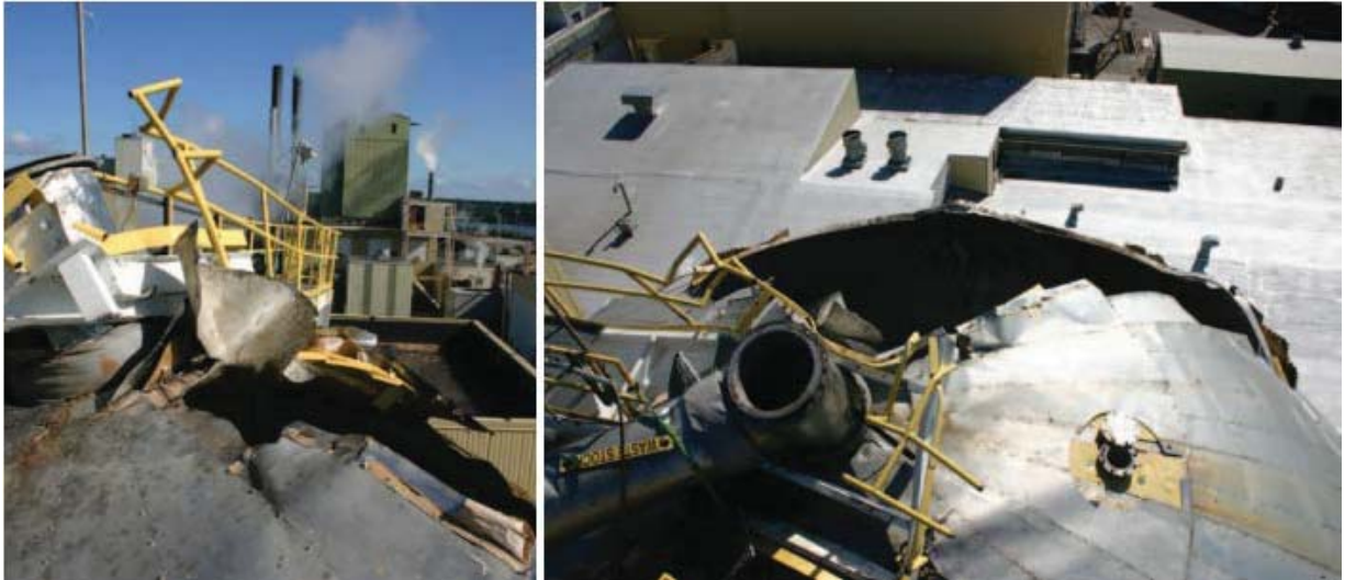
Figure 40. Post-Incident Photographs from the PCA Tomahawk Mill. These photographs show views of the top of the storage tank involved in the 2008 explosion at the PCA Tomahawk mill. Photograph: CSB.
