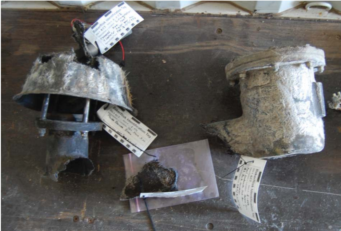
Figure 24. Post-Incident Pressure Vacuum Breaker. The foul condensate tank’s pressure vacuum breaker is shown post-incident. Photograph: PCA.
