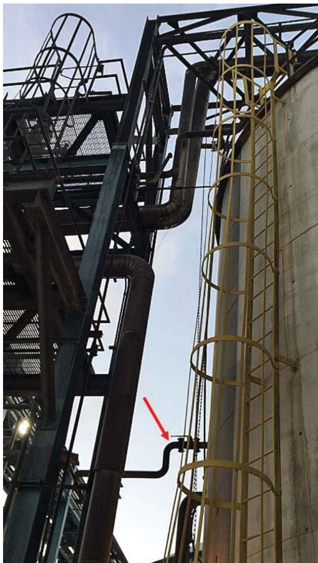
Figure 22. Pre-Incident Photograph of the Foul Condensate Tank. The line from the weir inside the tank to the turpentine recovery system is indicated by the red arrow. The valve at the foul condensate tank is kept open, but the valve at the turpentine recovery system ( Figure 21 ) is kept closed. Photograph: PCA.
