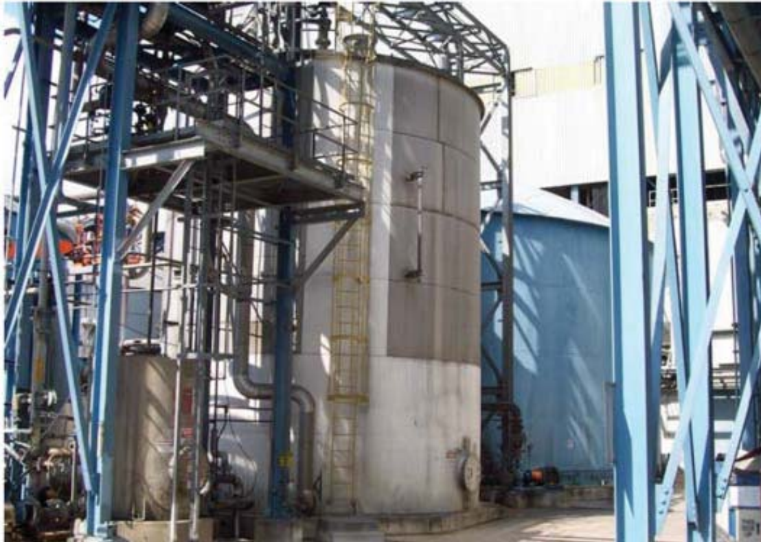
Figure 7. Pre-Incident Photograph of the DeRidder Mill Foul Condensate Tank. Welding work was being conducted above the tank on the pipe rack at the time of the incident. Photograph: PCA.
