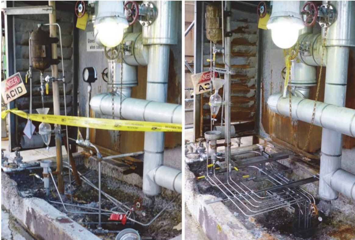
Figure 3. Photo showing the sulfuric acid sampling station at the Tesoro Martinez refinery. The photo on the left shows the sample station just after the February 12, 2014 incident and the photo on the right shows the sample station after repairs were made and the alkylolation unit was again operating. Workers informed the CSB that the concrete containment area, clearly visible in the photos above, had badly deteriorated from routine exposure to sulfuric acid.
