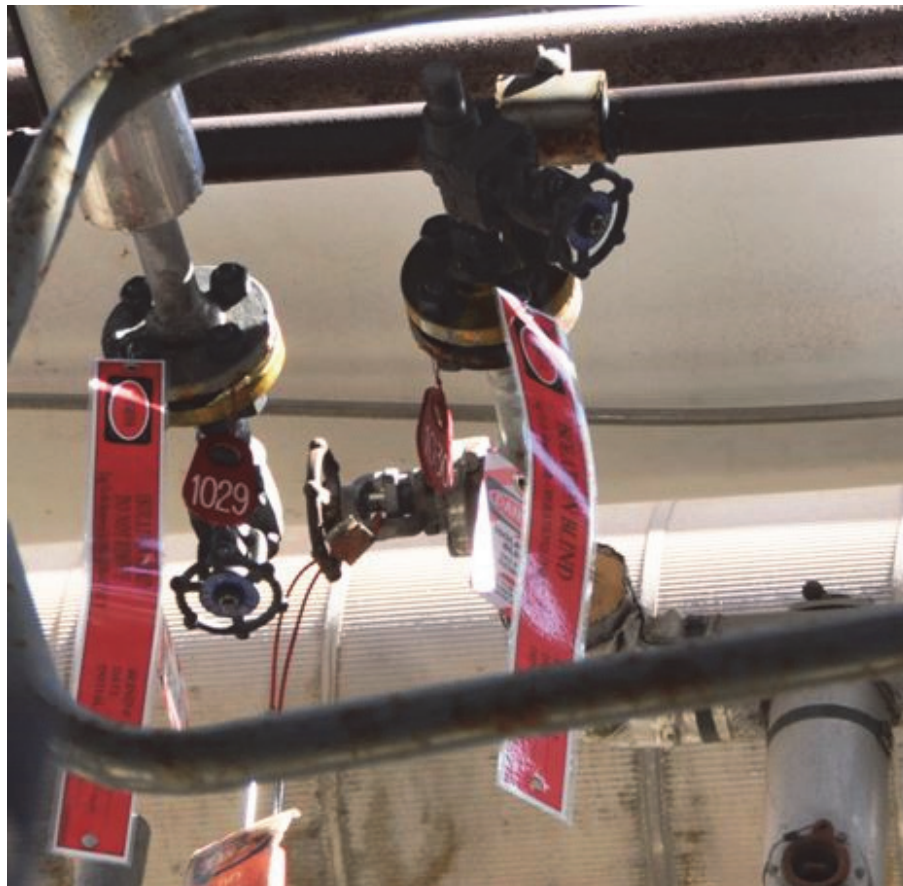
Figure 19. Photo of post-incident isolation of liquid butane supply piping to alkylation reactor. This photo shows the same piping shown in the right photo of Figure 18. Two days after the March incident, Tesoro modified the liquid butane isolation to match the API recommend practice, Tesoro’s corporate standards requirement, and Tesoro Martinez procedure recommendations by disconnecting and installing isolation flanges on each end of the isolated piping.
