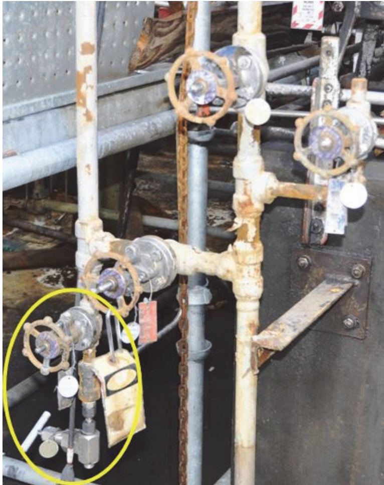
Figure 16. Photo of drain piping and valves. Evaluation of this equipment after the incident identified plugging in these piping components that prevented liquid from freely draining through the open valves.
