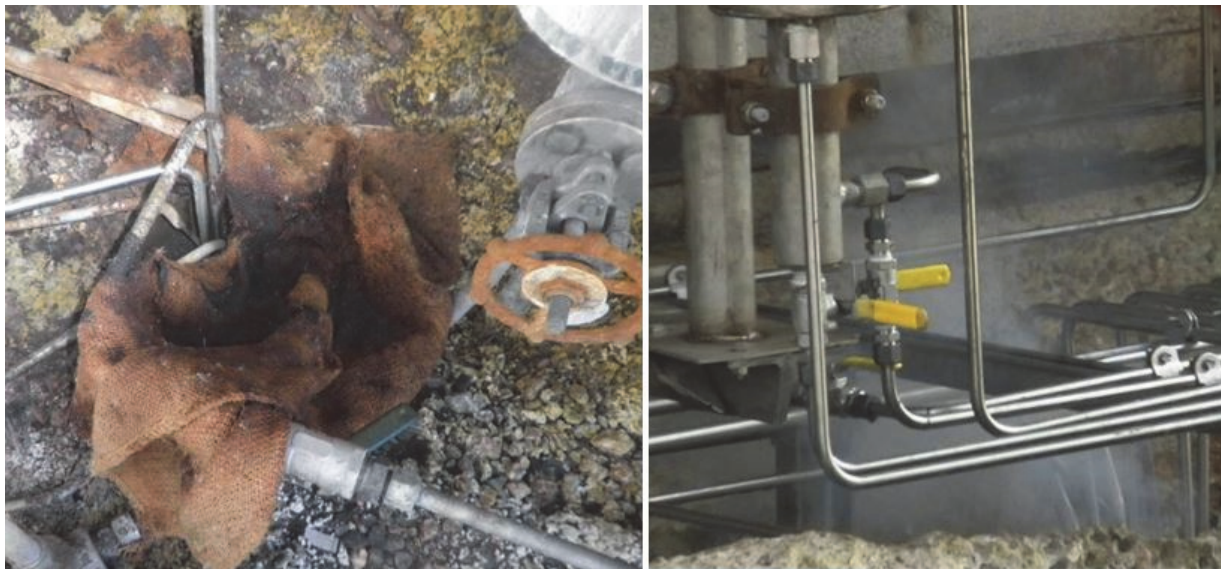
Figure 5. The photo on the left shows a burlap bag covering the process sewer drain at one of the Tesoro Martinez refinery sulfuric acid sample stations. The photo on the right shows the white vapor cloud released from the process sewer drain when Tesoro operators conduct the procedure to sample the sulfuric acid.
