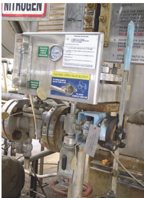
Figure 8. Photo showing one of the upgraded sample stations that Tesoro installed to reduce operator exposure to acid during sampling. Tesoro never resolved the reliability issues with these sample stations and the sample stations were taken out of service. As a result, they were not in use at the time of the February 12, 2014 incident.
