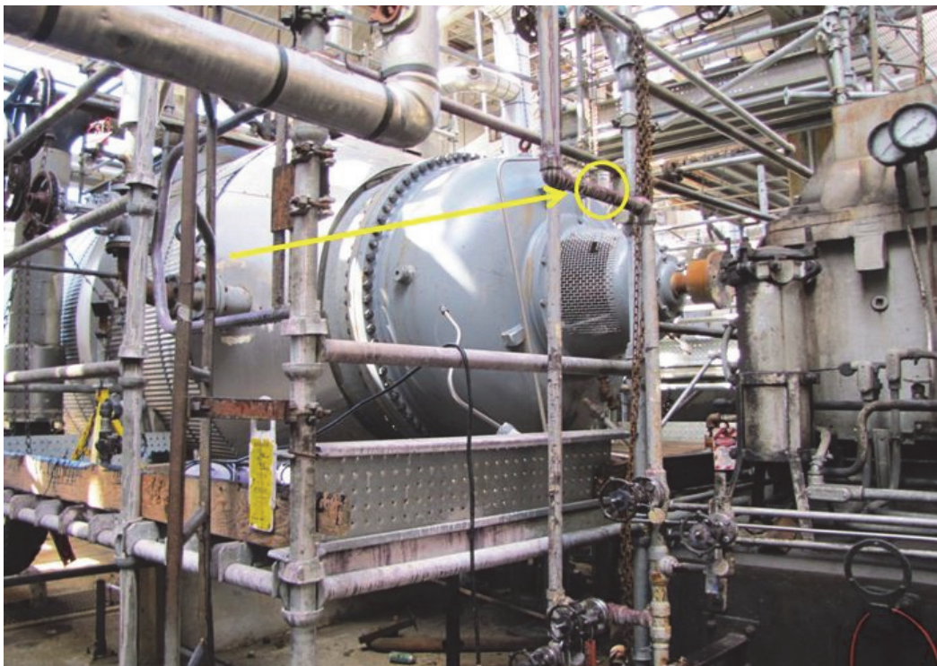
Figure 14. Photo of location of the March 10, 2014 incident. As depicted in Figure 12, two workers were located on this temporary scaffold platform and were cutting the piping (yellow circle) with a portable band saw.
