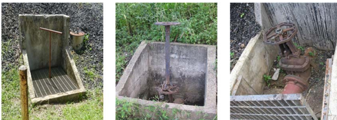
Figure 15: Various dike drain valves at CAPECO. Tank 409 fixed stem dike drain valve (left): position of the valve is undeterminable without physically turning the valve. Rising stem valves (center, right). In some cases, the valve position is hidden in the sump (center).
