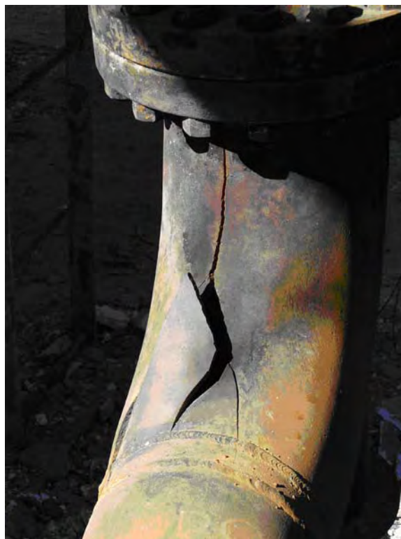
Figure 6. Crack in the 10" diameter propane mix control station inlet elbow
