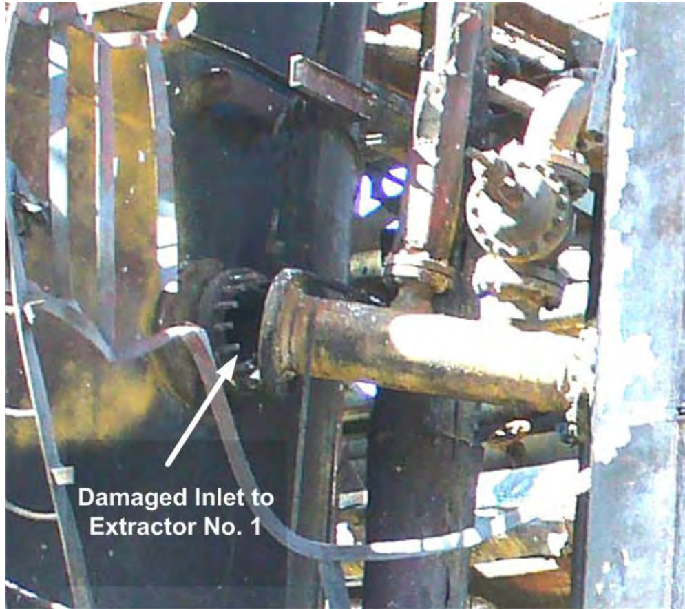
Figure 8. Damaged 10" propane inlet on Extractor No. 1
