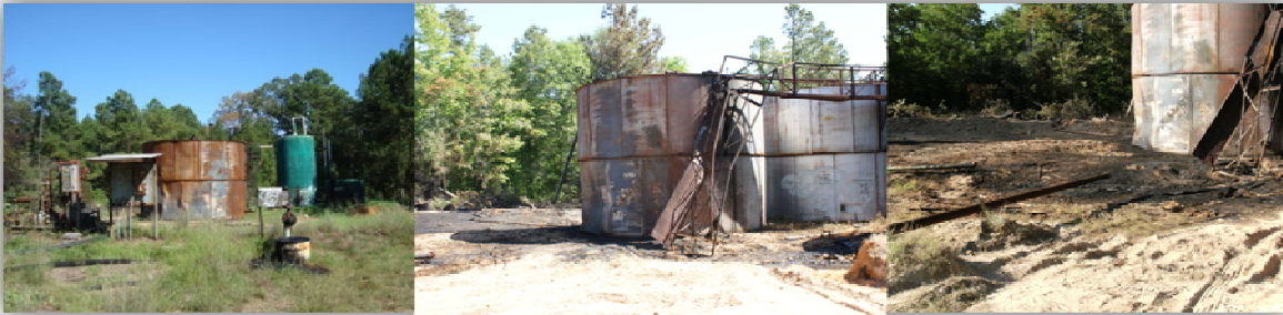
Figure 6-8: MC Production Oil tank site, New London, Texas
