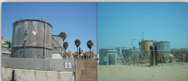
Figure 8-2: Tank battery in Los Angeles, California
