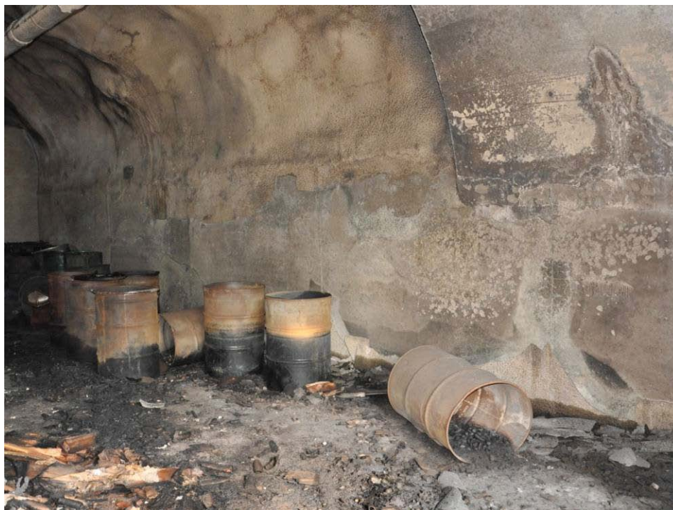
Figure 16. Interior of the magazine post-incident
