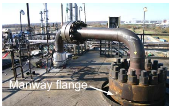
Figure 2. Pipe assembly connects 12-inch diameter process pipe to the reactor top manway (photo taken after the incident).
