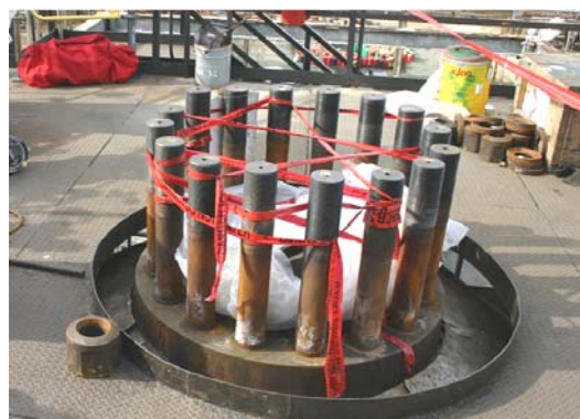
Figure 1. Plastic sheet and plywood disk on R1 manway. Red "danger" tape on the studs alerted workers of the unsecured confined space access opening.
