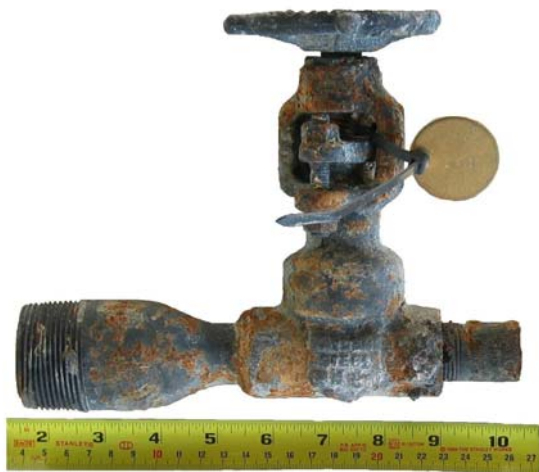
Figure 4. Valve and pipe.
