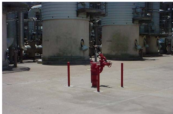
Figure 9. Protection of fire fighting equipment.
