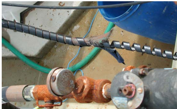
Figure 2. Failed stainless-steel transfer hose.
