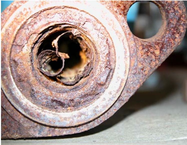
Figure 25. Corrosion buildup in chlorine repackaging piping system.
