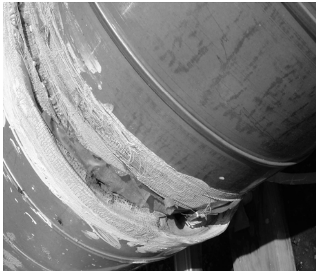
Figure 9. Condition of duct tape used to seal gaps.
