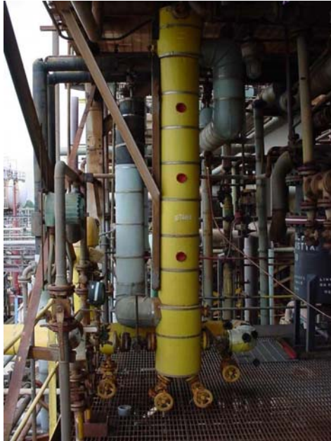
Figure 3. Vertical chlorine cooler in G-143a process.
