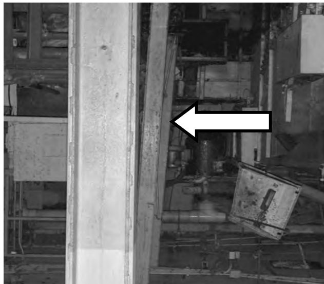
Figure 8. Bent support column in line 401 blend room.
