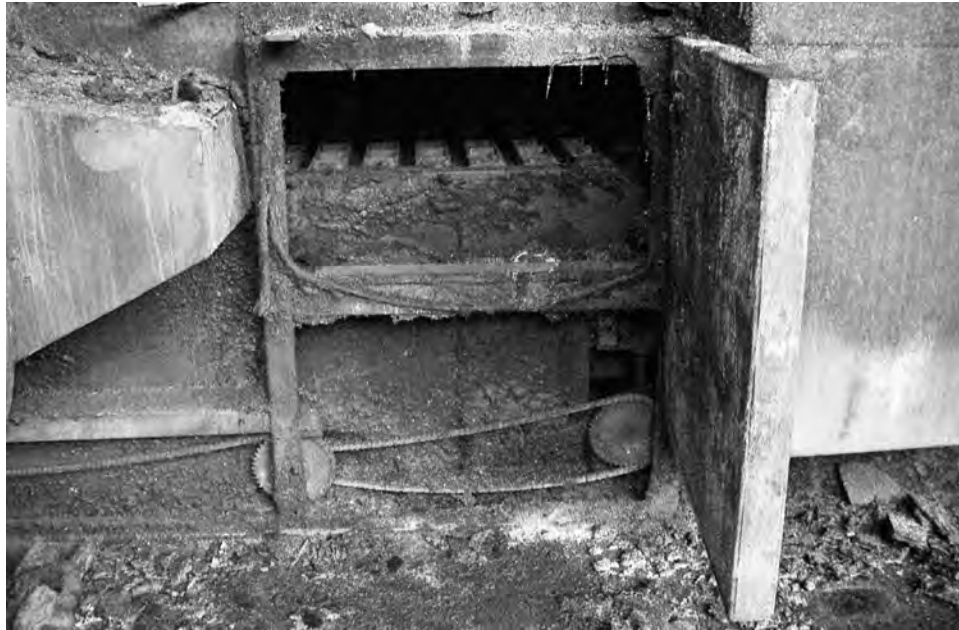
Figure 13. Interior of line 405 oven.
