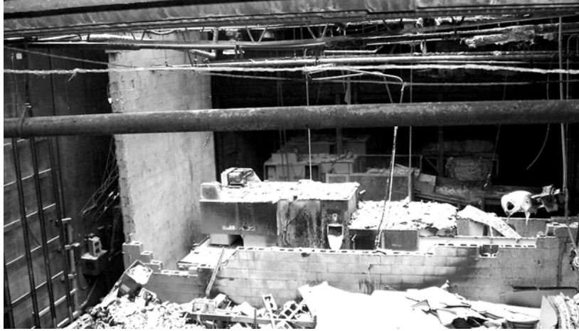
Figure 7. Collapsed firewall between lines 403 and 405.
