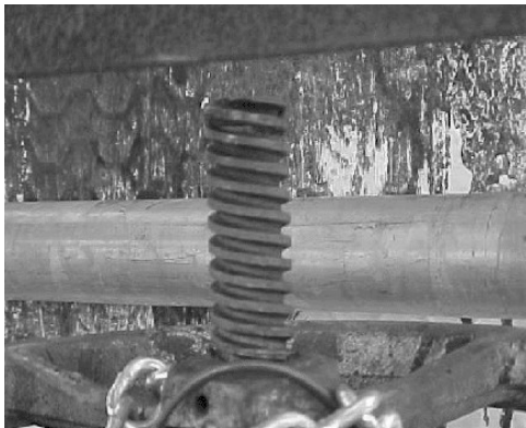
Figure 5. Closeup of stem of block valve (C), upstream of LCV-150, with the valve wheel fully tightened.
