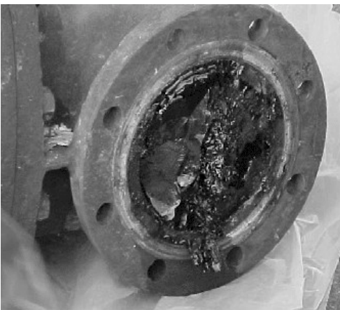
Figure 3. Closeup of material blockage of block valve (C), upstream of LCV-150.
