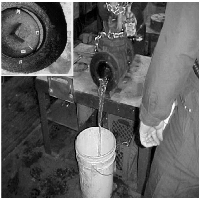
Figure 7. Leak test of the naphtha stripper level control bypass valve (B) in the closed position, showing significant water flow.
