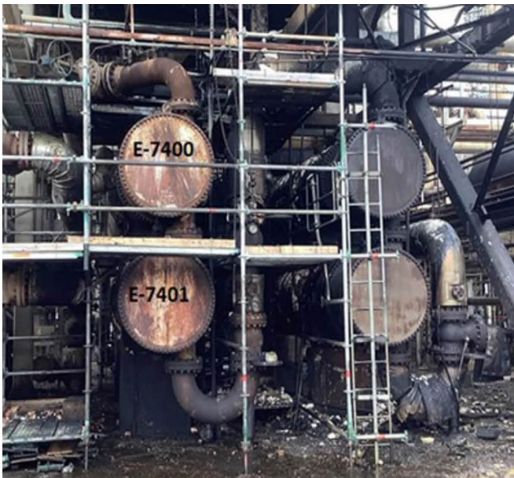
Figure 1. Heat exchangers after the incident. (Credit: Pemex)
