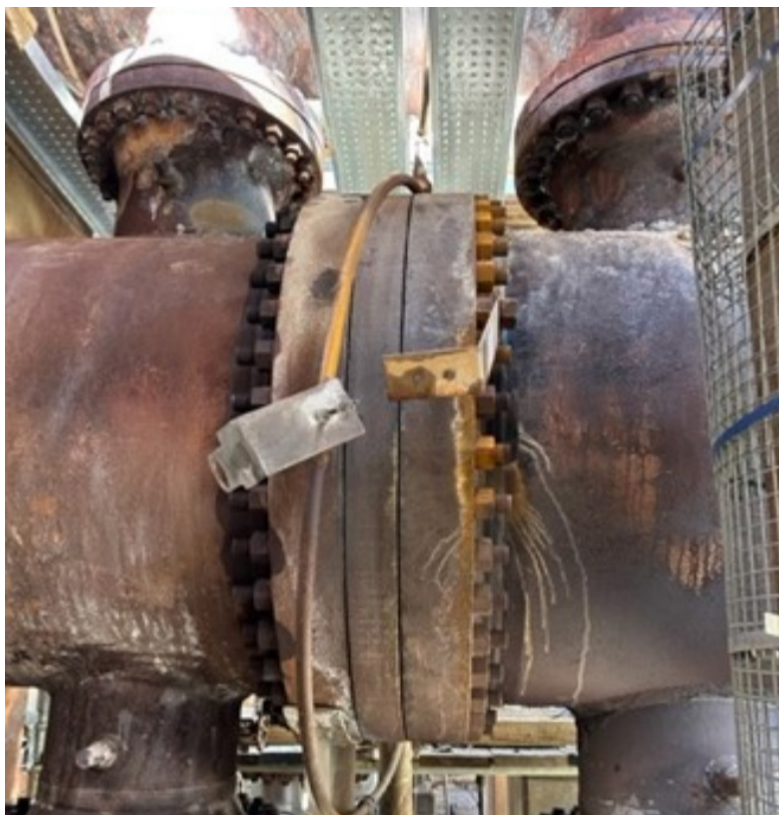
Figure 1. The Flange Where the Leak Occurred. (Credit: CITGO)
