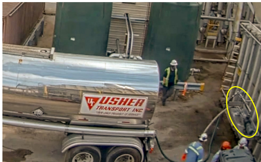
Figure 1. Caustic Unloading Pump (yellow oval). (Credit: Georgia-Pacific)
