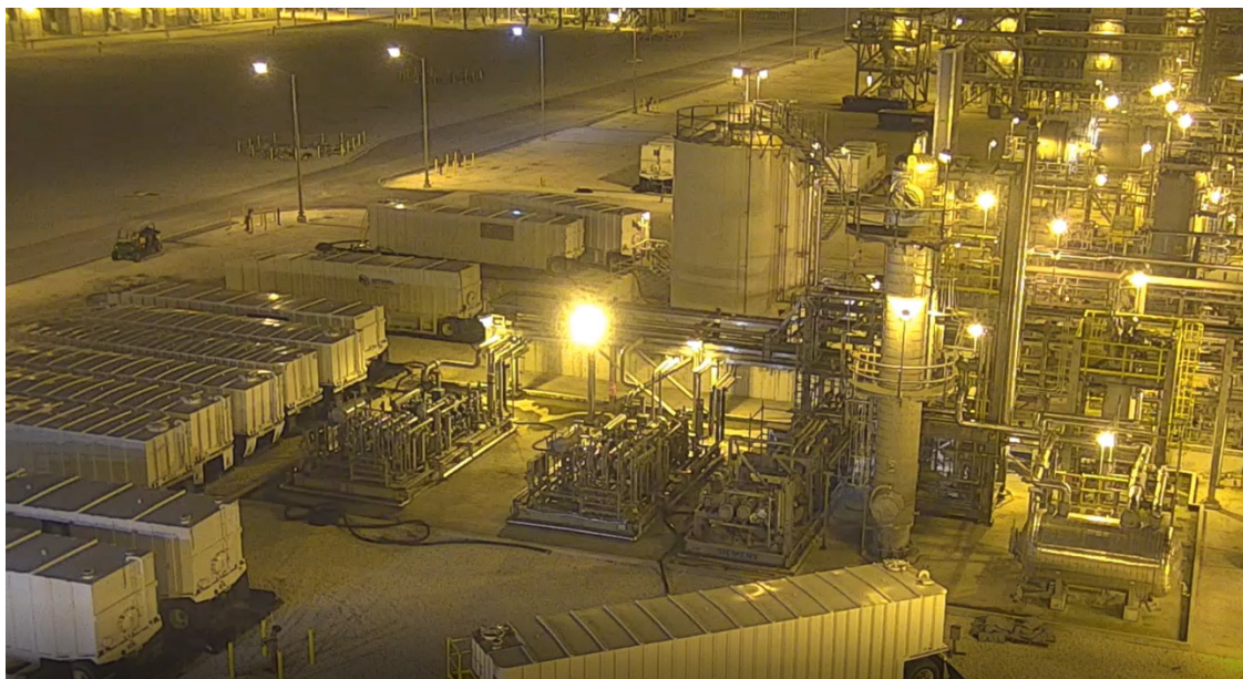
Figure 1. Spent Caustic Storage and Handling Equipment at the LACC Facility. (Credit: LACC)
