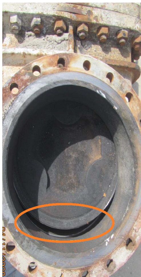
Figure 2. Nearly closed outlet valve. (Credit: Valero Meraux Refinery, modified by CSB)
