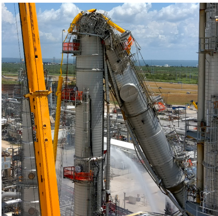
Figure 1. Collapsed Distillation Tower at BTP. (Credit: BTP)
