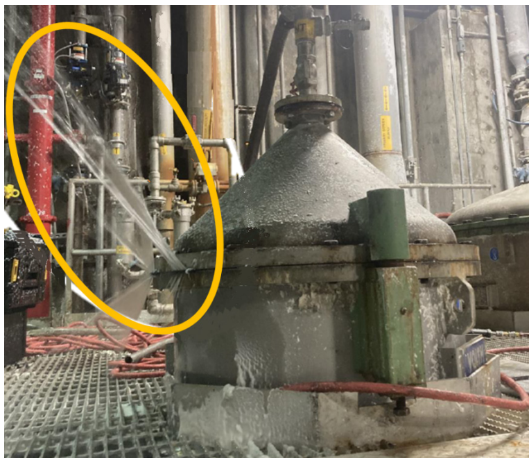
Figure 1. Hot water and pulp sprayed out of the pulp screen. (Credit: Georgia-Pacific)
