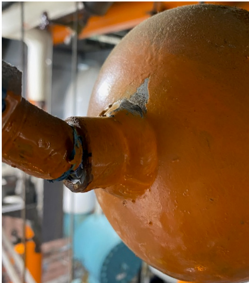
Figure 1. Damaged Ammonia Piping. (Credit: HMF)
