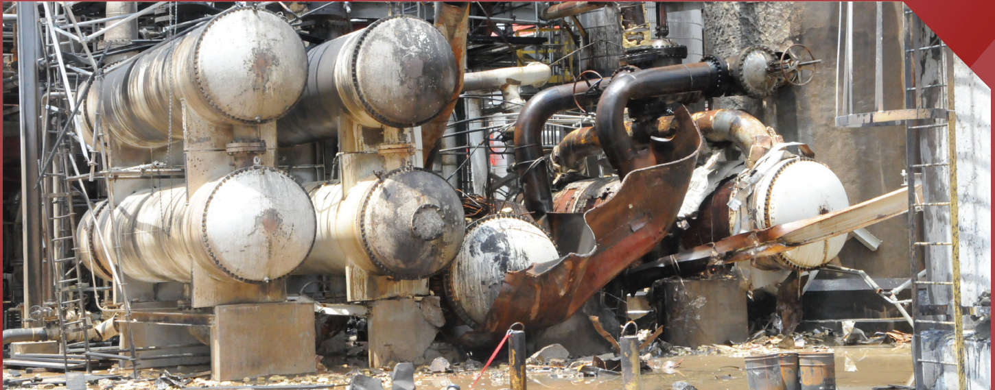
View of the damaged heat exchanger at the Williams Olefins Plant.
