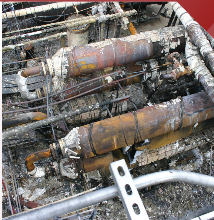
Aerial view of heat exchangers damaged from the Tesoro Refinery explosion and fire.
