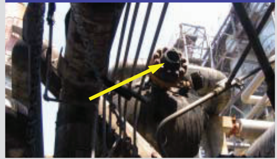
Figure 1. Carbon steel RHU heat exchanger outlet pipe (arrow) ruptured after operating only 3 months in high-temperature hydrogen service.
