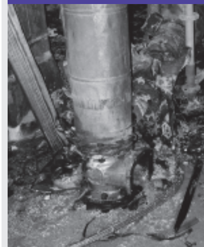
● Figure 1. Ruptured pipe/valve and fire damage.
