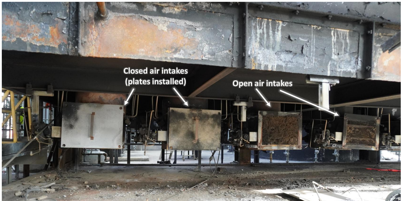
Figure 9. Post-incident as-found condition of the air side of four of the burners. (Credit: CSB)
