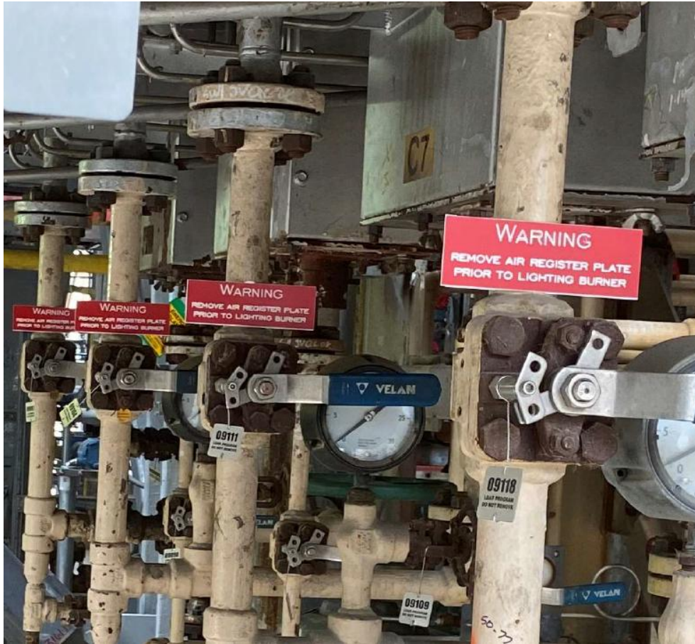
Figure 25. Signage installed at burner fuel gas valves at the Marathon Martinez facility post-incident. (Credit: Marathon)
