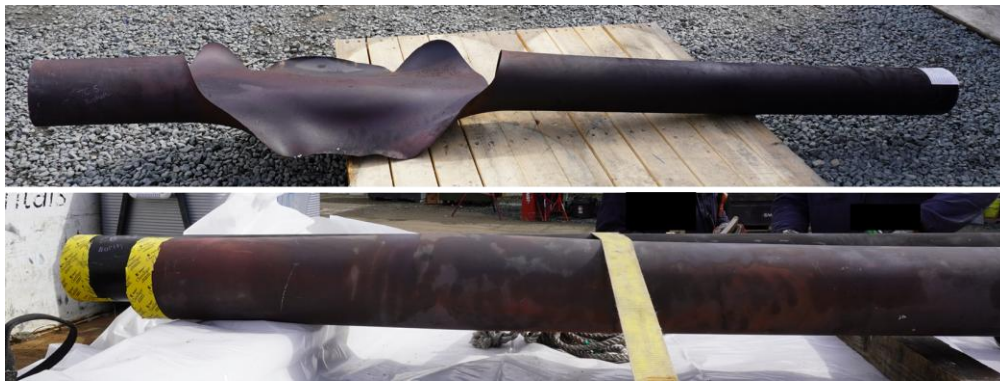
Figure 18. Convection section tubes showing more than 3% outer diameter growth. (Credit: CSB)
