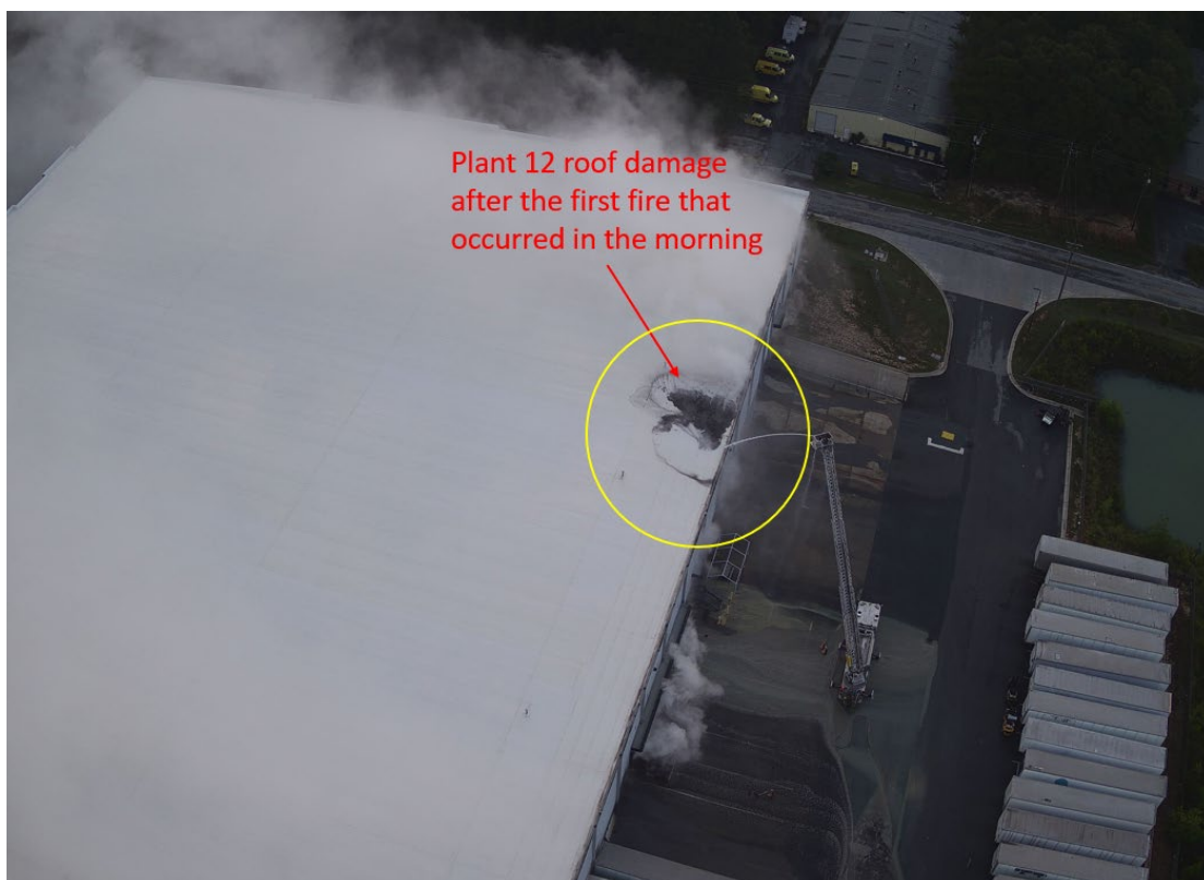
Figure 1. Plant 12 warehouse roof damage at approximately 8:10 a.m. after flames were extinguished (Credit: Rockdale County Fire Rescue)
