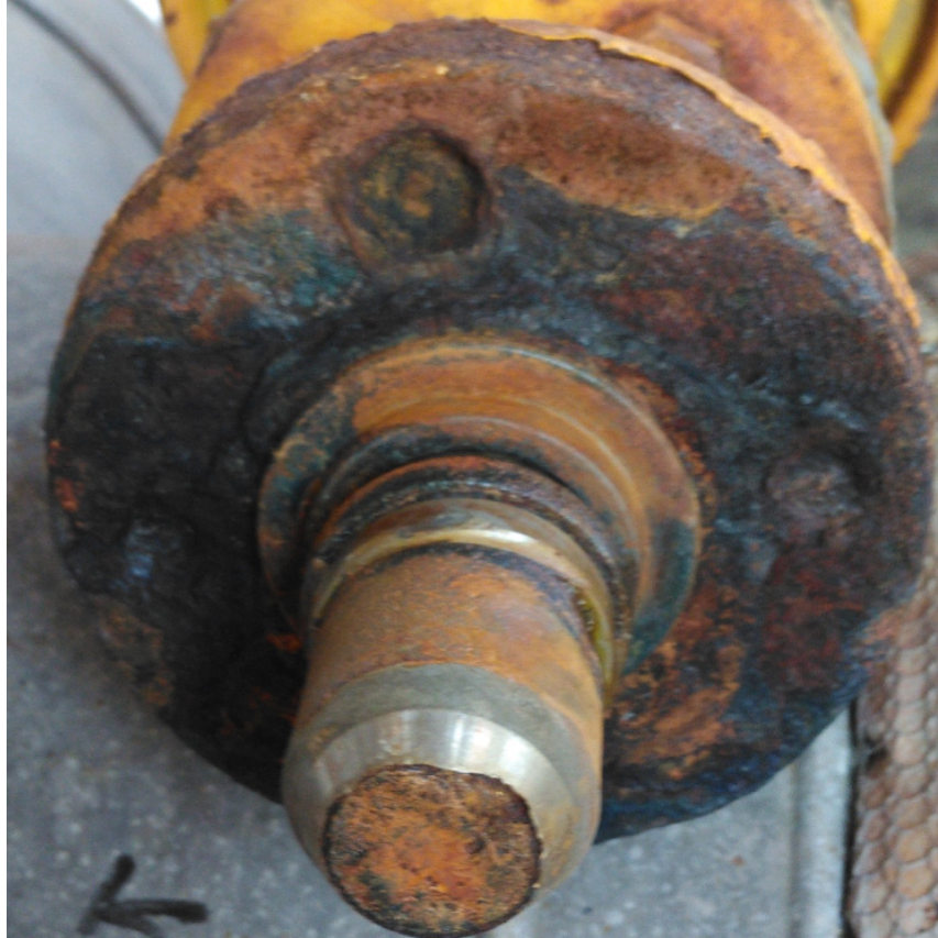
Figure 1. Corroded drain valve's bonnet and bolts. (Credit: BASF)
