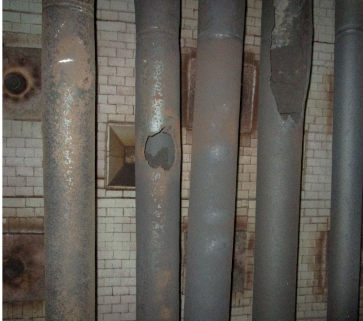
Figure 3. Failed fired heater tubes. (Credit: Chevron-Phillips)
