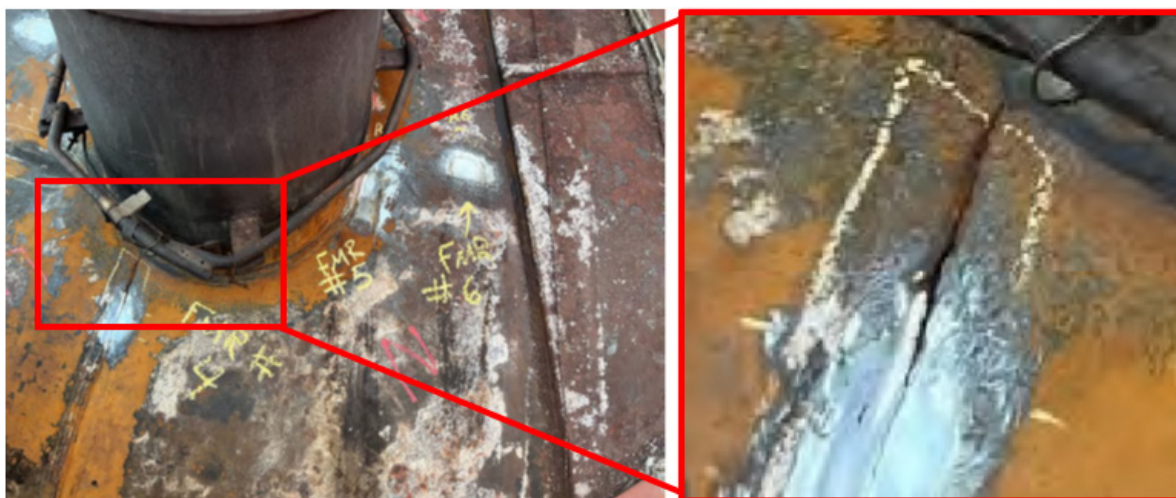
Figure 2. One of the cracks in the reactor’s head. (Credit: LyondellBasell, edited by the CSB)
