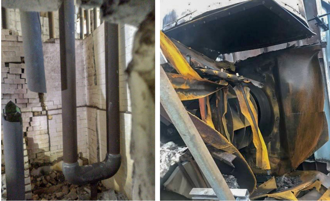
Figure 5. Fired heater explosion damage. The left image shows the broken tube and walls, and the right image shows a fan. (Credit: Chevron Phillips)
