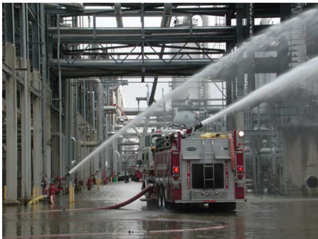
Figure 4. Photo included in the CSB Formosa Investigation Report. This photo shows Formosa Emergency Response Team equipment.
