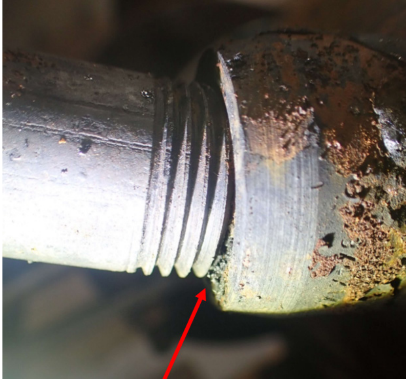
Figure 2. Damaged Mineral Oil Piping. (Credit: Chemtool)
