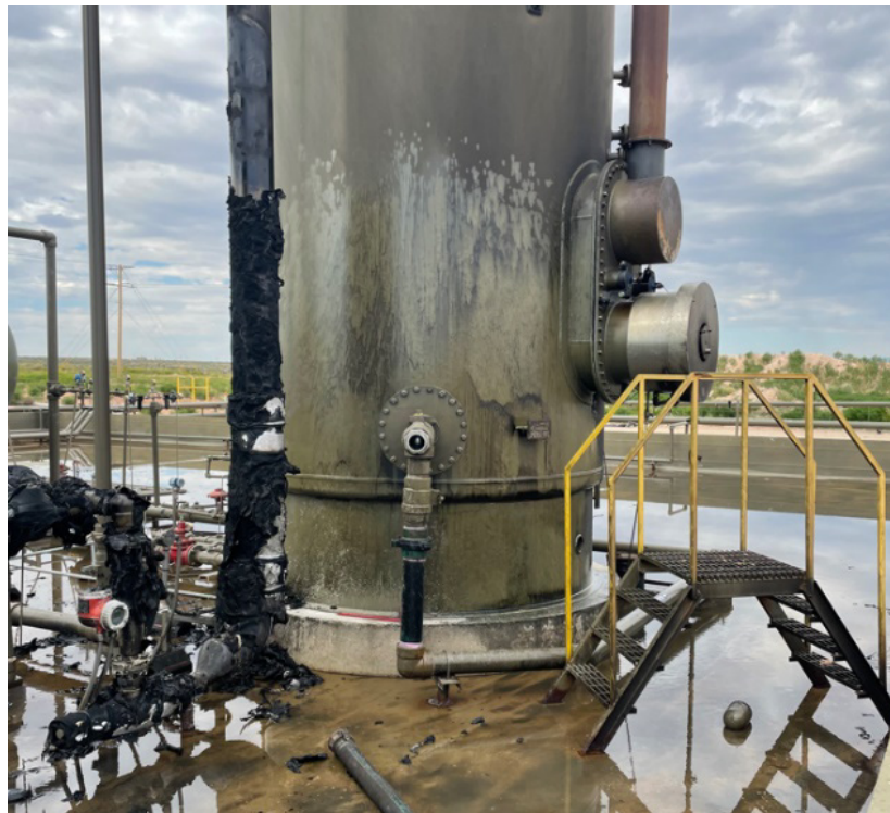
Figure 1. Damaged Heater Treater After the Fire at ConocoPhillips. (Credit: ConocoPhillips)
