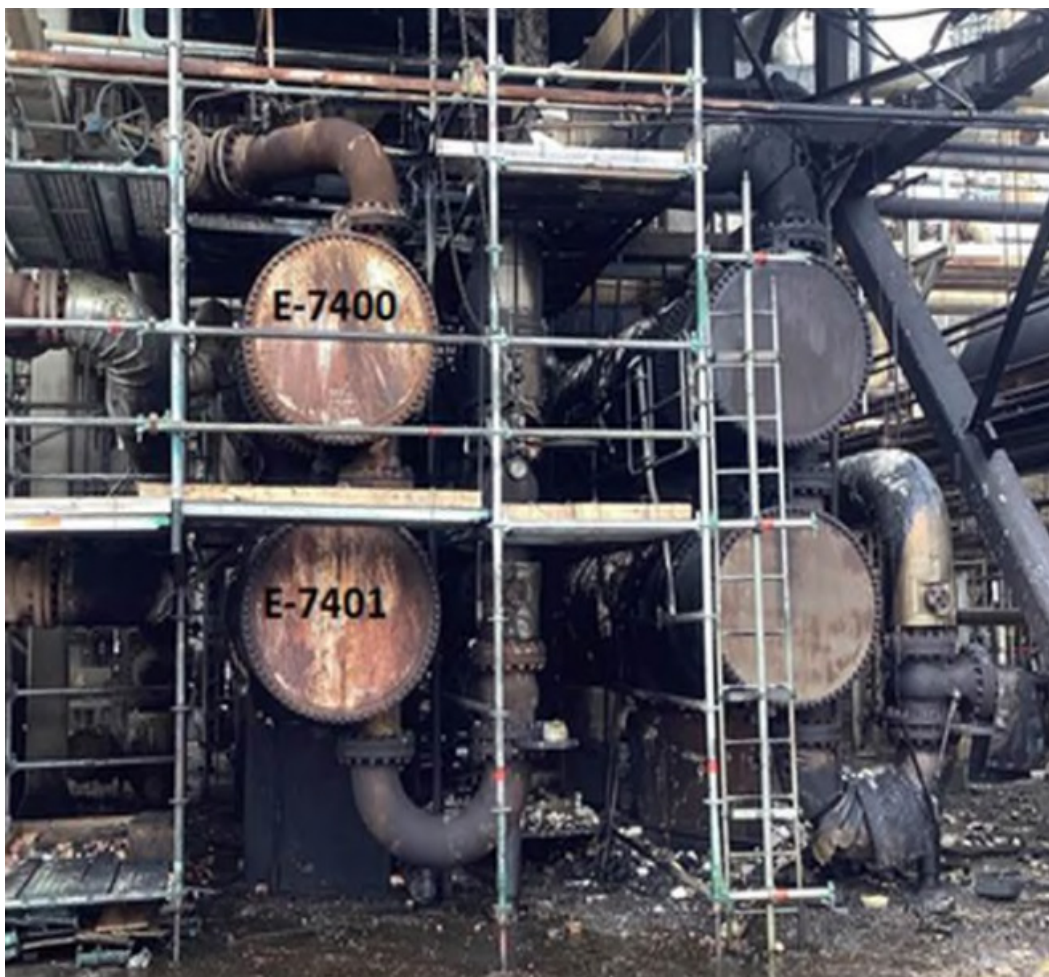
Figure 1. Heat exchangers after the incident. (Credit: Pemex)
