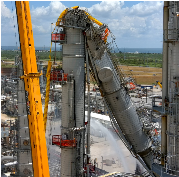
Figure 1. Collapsed Distillation Tower at BTP. (Credit: BTP)
