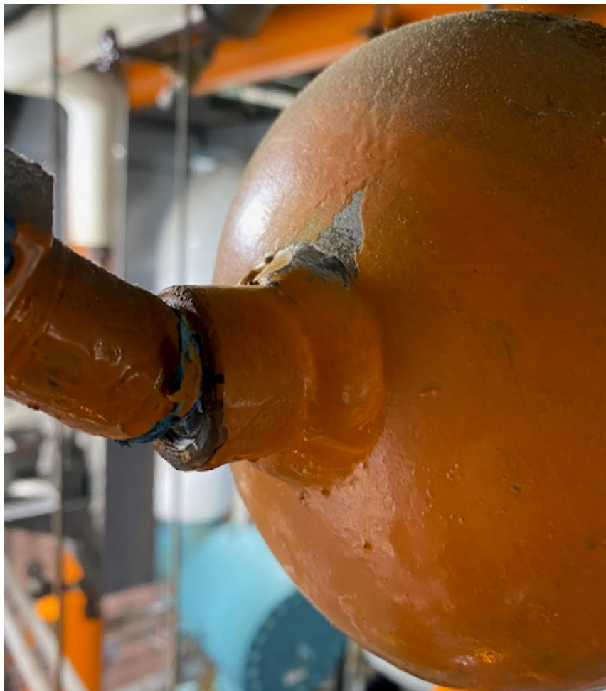
Figure 1. Damaged Ammonia Piping. (Credit: HMF)
