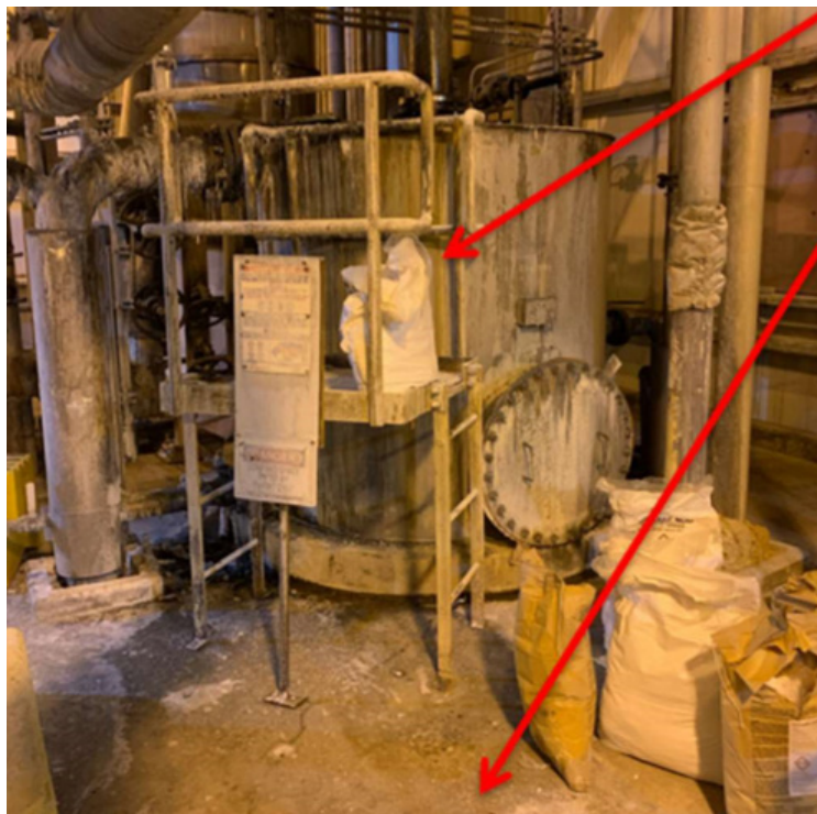
Figure 1. The Tank. The red arrows show the approximate locations of two of the operators. (Credit: Domtar)
