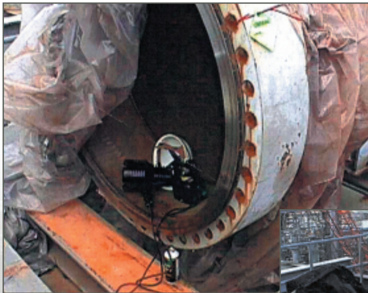
Large open pipe end where the two victims were working
