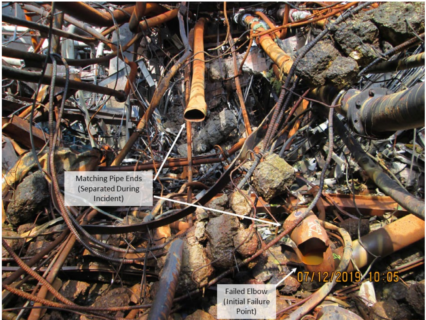
Figure 7. Photo of the ruptured pipe elbow found post-incident. (Credit: PES)
