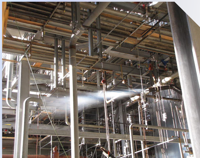
Photo of "gas blow" method which was used at Kleen Energy to remove debris from the piping.
