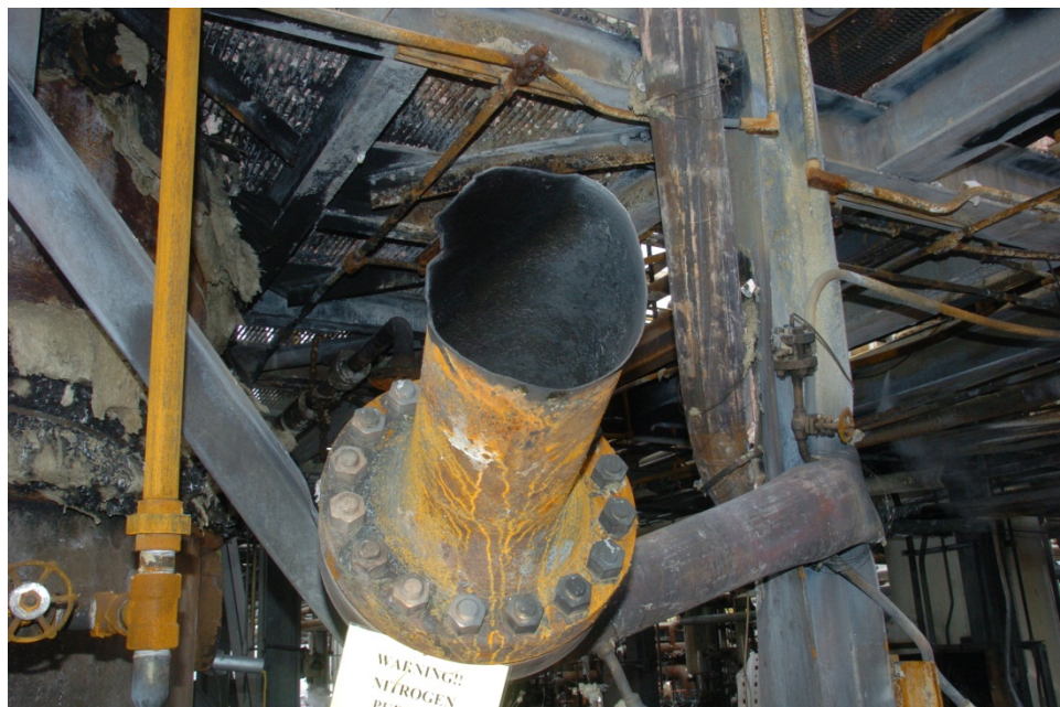
Figure 12. Ruptured end of pipe wrapped around support beam.
