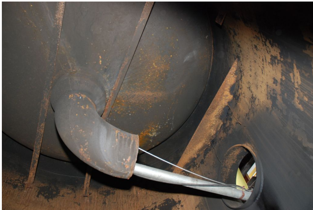
Figure 19. Images of the upstream end of the fractured pipe prior to its removal in March 2010.
