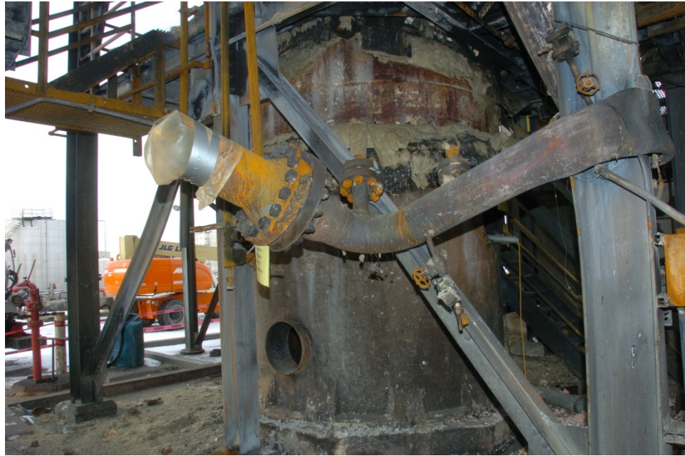
Figure 11. R30101 discharge pipe bent around reactor support beam.
