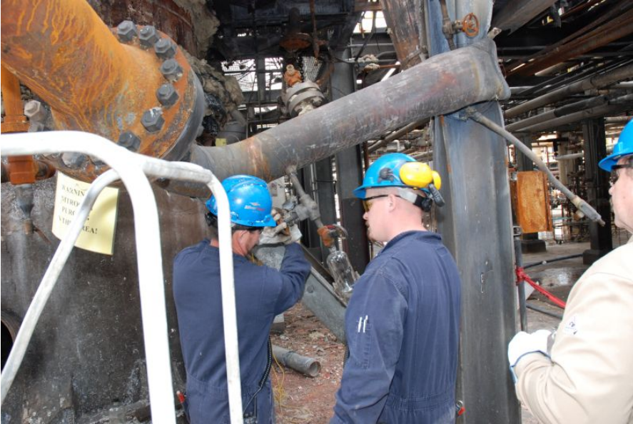
Figure 22. Image of SER employees draining fluid from the "SER 36" valve in March 2010.
