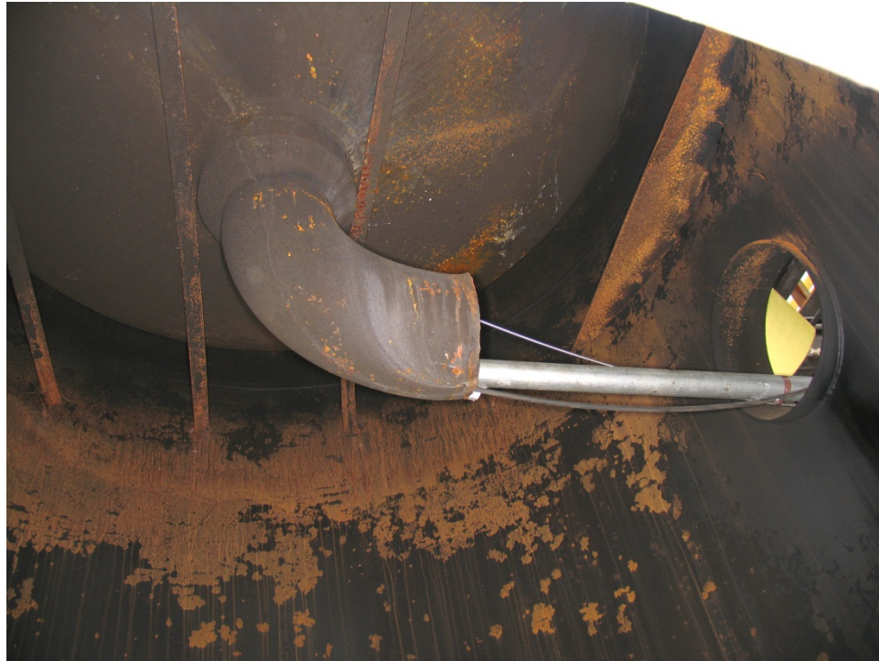
Figure 13. Ruptured end of pipe still attached to R30101.
