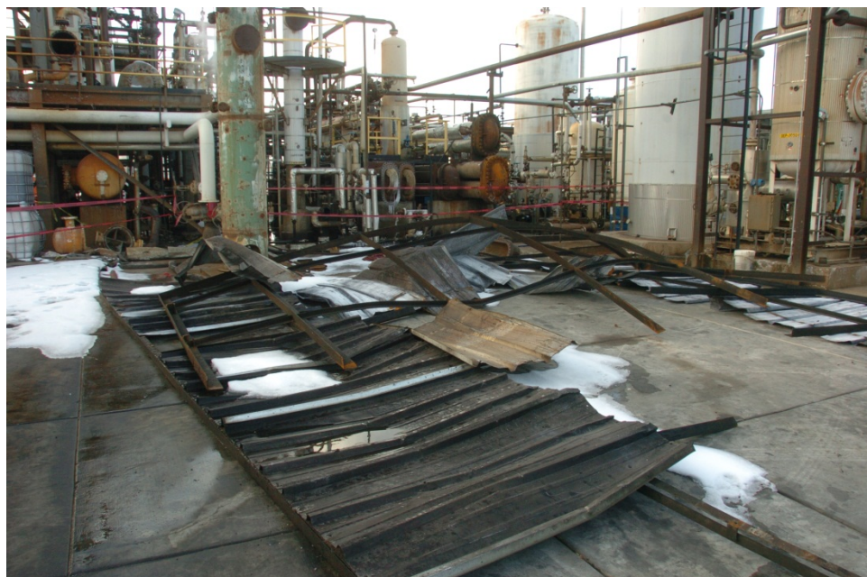
Figure 14. Explosion damage to light structural elements, hydro pad.
