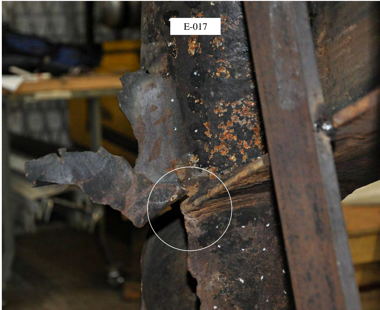
Figure 5 Photograph of the closest approach between the rupture and welded pipe guides of sample E-017. All other guide welds ended 4 to 6-inches from the rupture edge.
