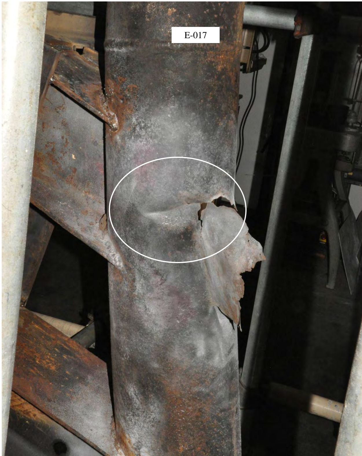
Figure 6 Photograph of the ruptured section of sample E-017. A small degree of buckling was present near the upstream welded pipe guide.
