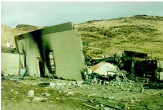
View of booster room 1 following the explosion, with west wall still standing. The five workers in this room survived.
