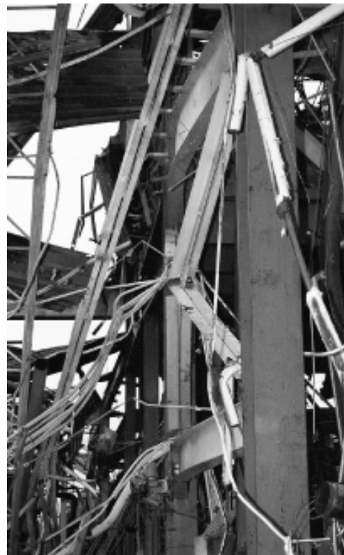
Figure B-1. Beam and cross bracing deflected southeastward toward warehouse.
