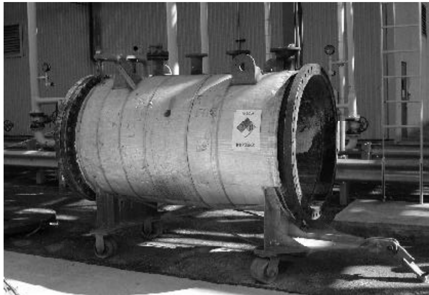
Figure 3. KD-502 polymer catch tank (actual vessel with one cover removed).
