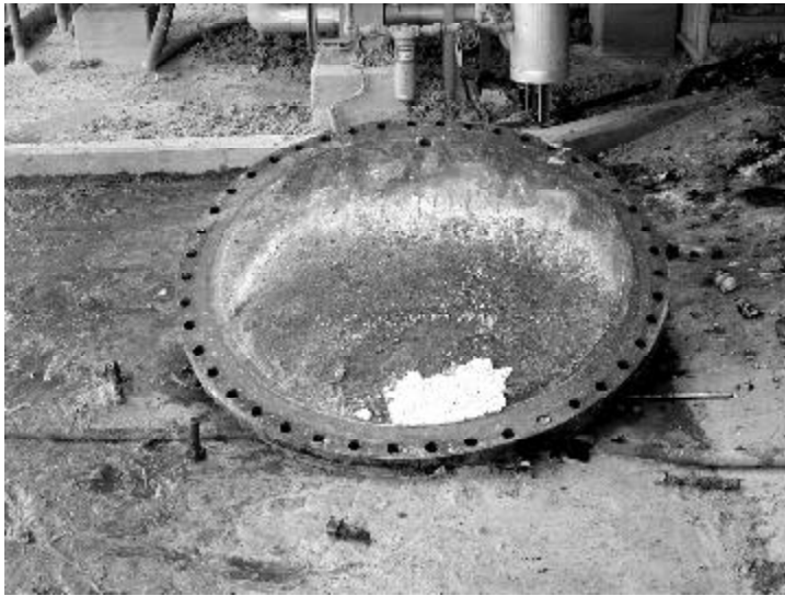
Figure 6. Polymer catch tank cover.
