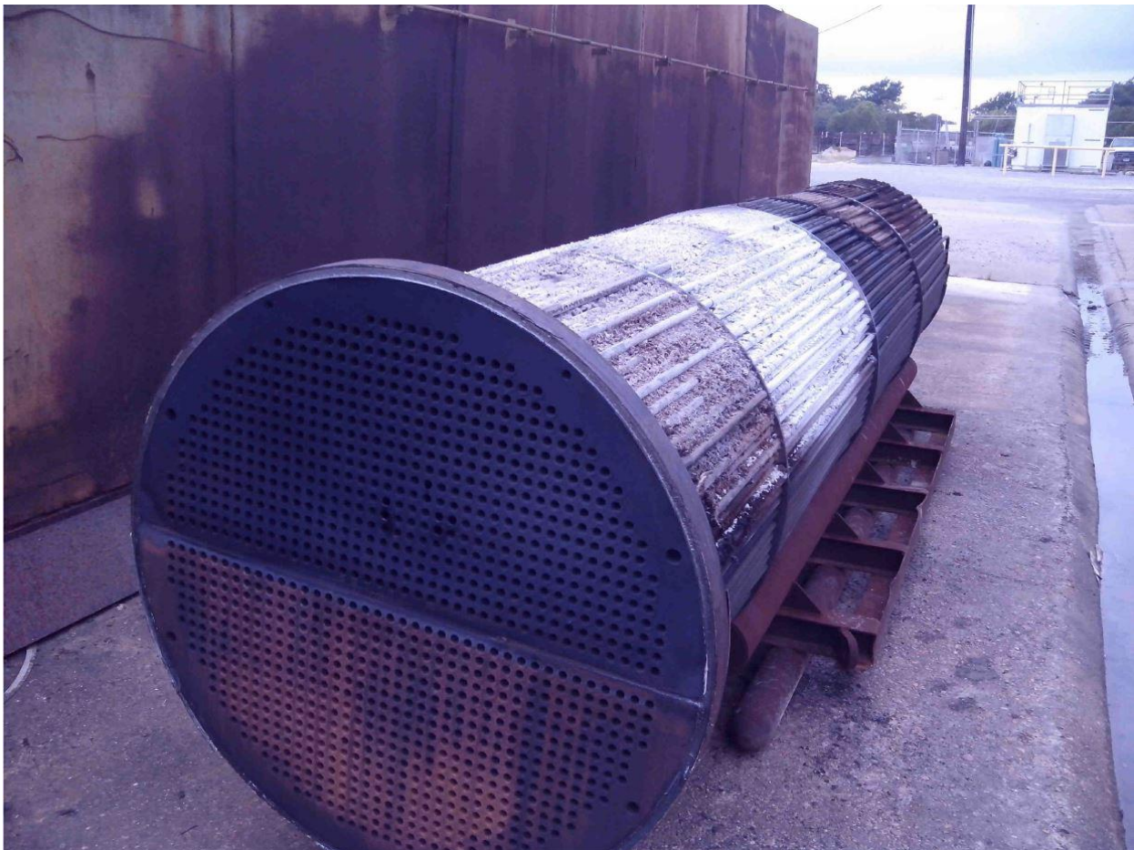
Figure 12. Polymer found on methyl acetylene removal tower reboiler bundle pulled on or around September 10, 2019. (Credit: TPC)
